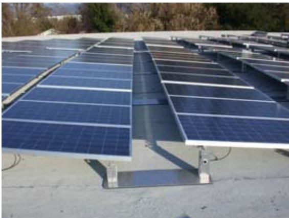
Fig. 4-1. The free-standing (FS) system developed under this contract is the flagship PV array mounting system offered by the company.
