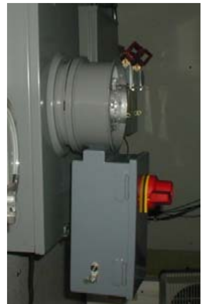
Fig. 2-20. The MID installed in a ringless style meter base.
