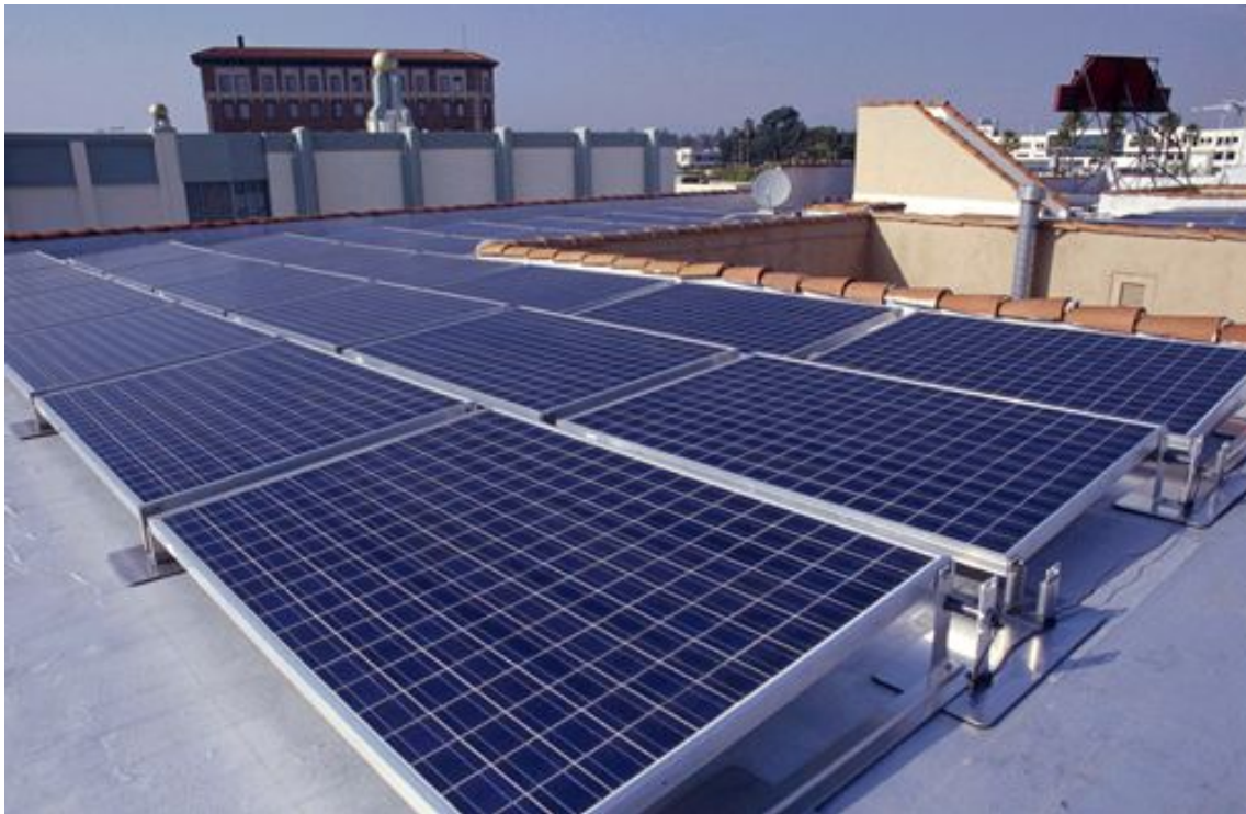
Fig. 4-9. An example FS installation with the original hardware.
