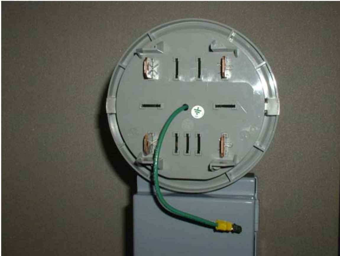
Fig. 2-5. A jumper through the back of the meter extender carries the equipment ground from the enclosure. This ground wire is shown with a spade terminal. A free length of wire with a mating spade terminal would be secured to the neutral lug in the meter socket.
