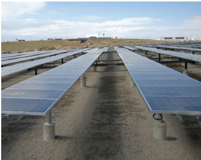
Denver, a Solar America City, installed a 2-megawatt PV system at Denver International Airport.
