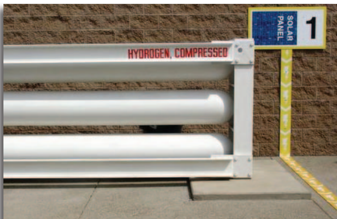
Compressed hydrogen storage tanks at the SMUD solar-powered hydrogen vehicle fueling station in Sacramento, California.
