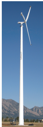
Entegriy EW50 (50 kW) on tubular tower.
