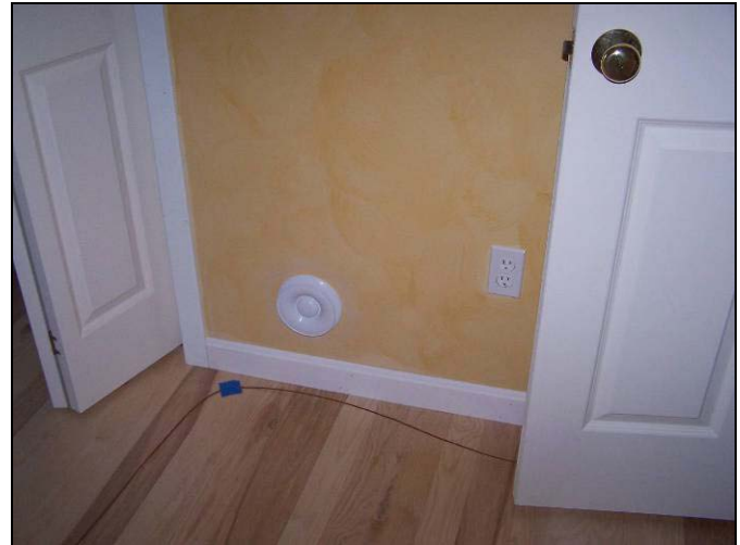
Figure 10. Second floor southeast bedroom diffuser
