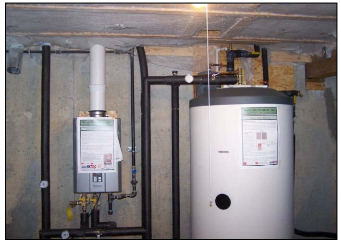
Figure 6. Basement northeast corner domestic hot water setup
