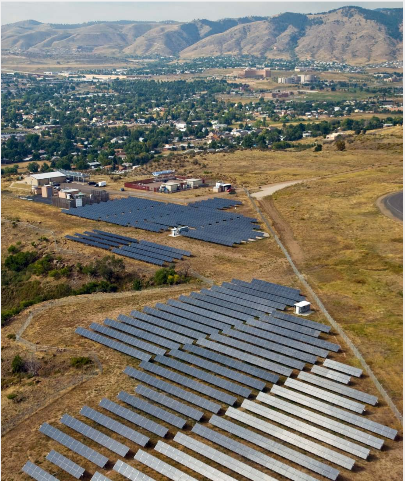
NREL's new Mesa Top Photovoltaic Array will provide more than 7% of NREL's annual electricity needs.
