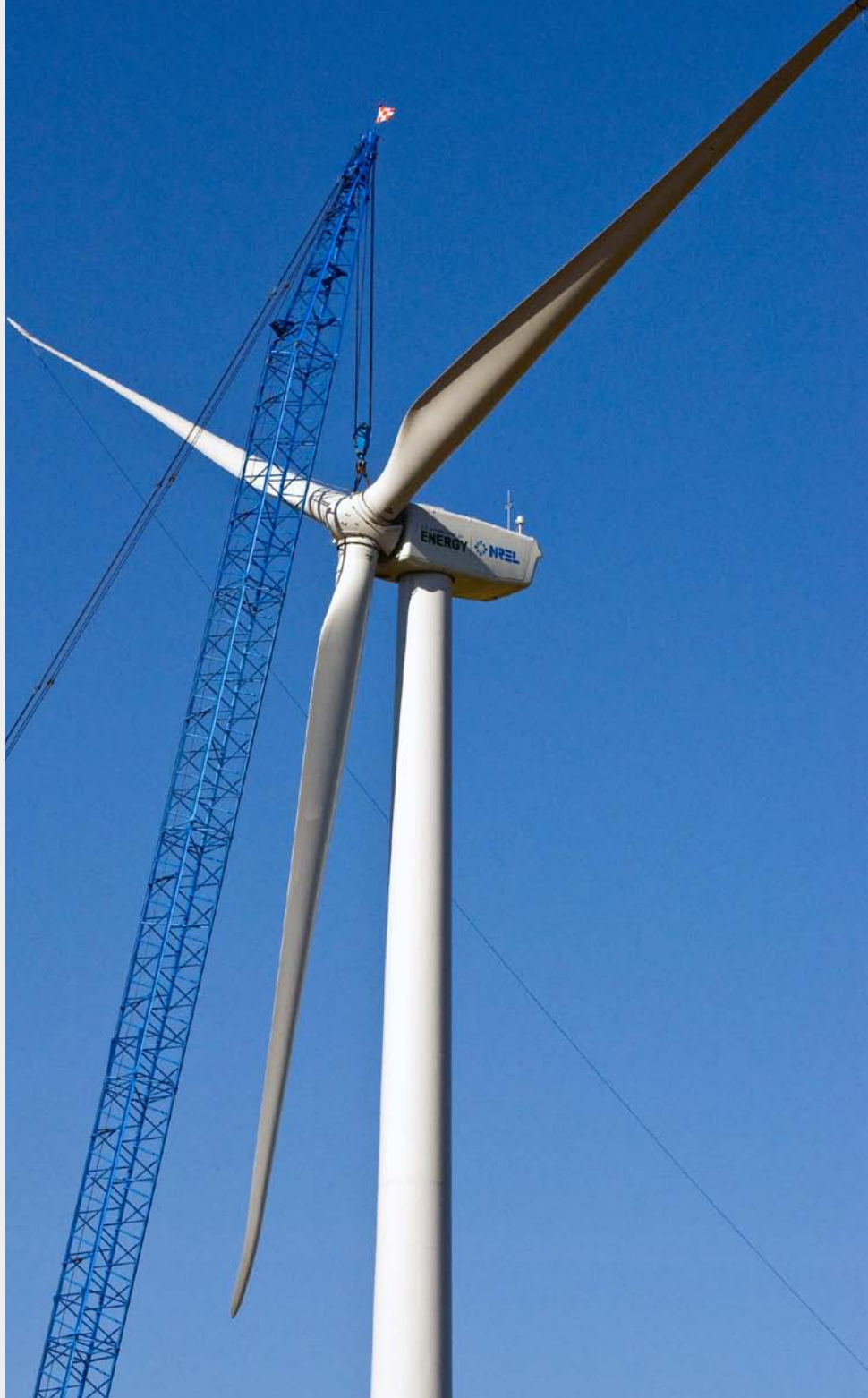
This 1.5-megawatt General Electric wind turbine, purchased for NREL by DOE, was one of two large wind turbines installed at NREL in FY 2009.
