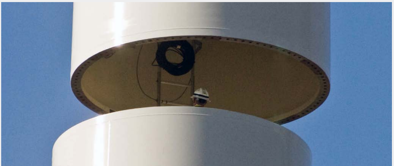
The large scale of the new NREL wind turbines is demonstrated by this worker, who is helping to guide two parts of the tower together as the top part is lowered by a crane.
