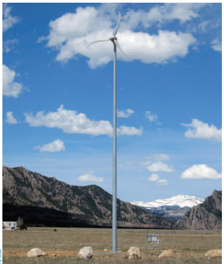
The Southwest Windpower Skystream 3.7 wind turbine rated at 2.4 kW, with a blade diameter of 3.7 meters, and mounted on a 10-meter monopole.
