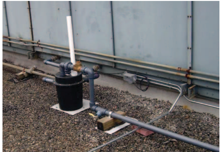
Initial piping and the condensate collector next to one air handler unit
