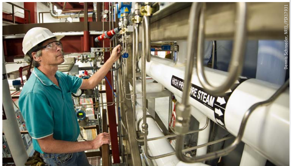
Master technician and pilot plant operator Robert Lyons inspects the high-solids pretreatment reactor in the Integrated Biorefinery Research Facility. The new reactor greatly enhances NREL's pretreatment testing and process development capabilities.
