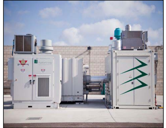
Figure: 9 FuelCell Energy unit installed at Gills Onions. Photo Courtesy of Gills Onions
