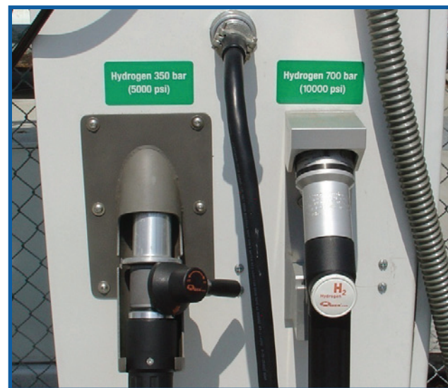
Burbank, CA station. Photo: NREL
