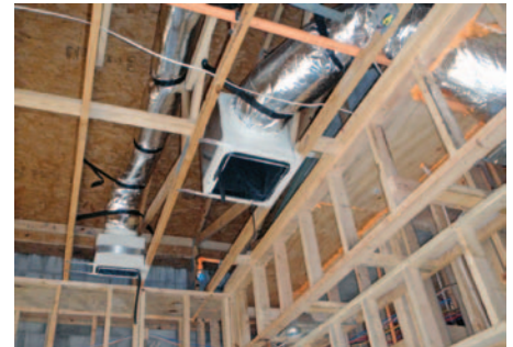
All ductwork is within the conditioned space and well-sealed using mastic.
