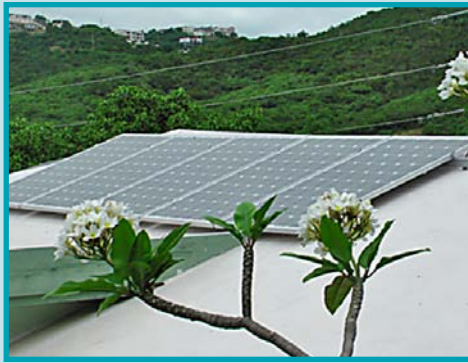
PV panels installed at the Montessori School on St. Thomas. Photo from Don Buchanan, Virgin Islands Energy Office
