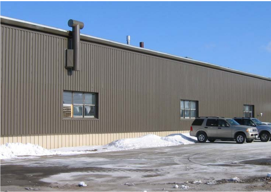
Transpired collector mounted on the south wall of the building. Photo by Ed Hancock, NREL/PIX 19363
