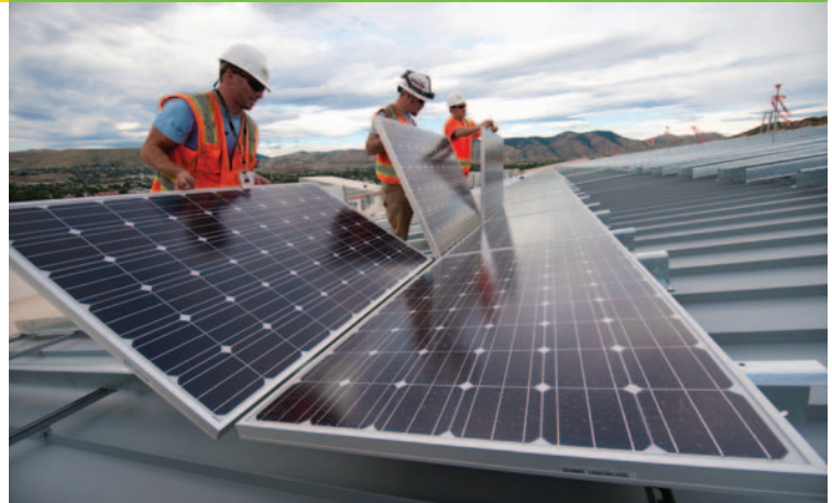
PV panels being installed on the roof of the Research Support Facility (RSF) at the National Renewable Energy Laboratory in Golden, Colorado. Photo by Dennis Schroeder, NREL/PIX 17843
