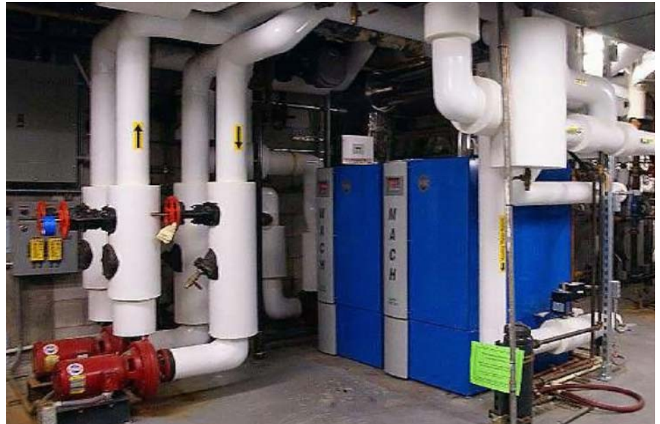
Engineered sites received boiler assessments and upgrades as part of the BLM ESPC.
