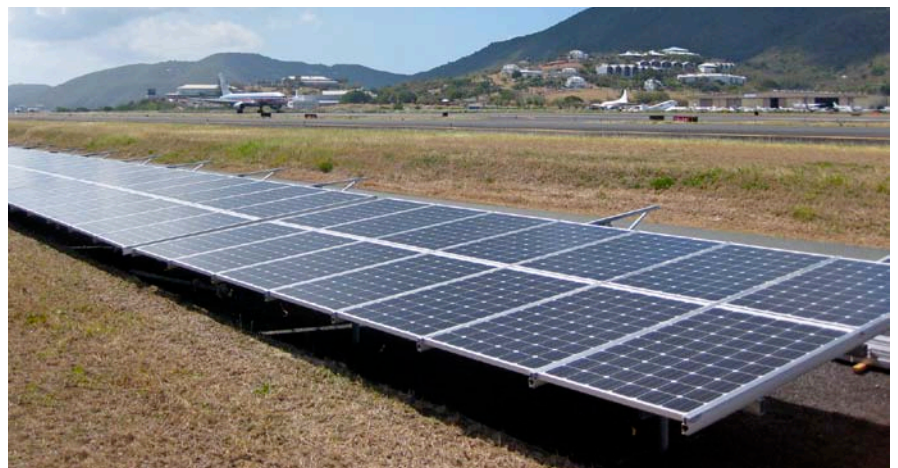
The first thing visitors see upon landing in St. Thomas is the VI Port Authority’s newly installed 450-kW PV system flanking the runway at Cyril E. King Airport. NREL/PIX 18953
