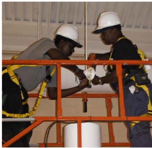
Energy Systems Group workers replace old lights with energy-efficient ones at Yvonne E. Milliner-Bowsky Elementary School on St. Thomas. Photo from Don Buchanan, VI Energy Office
