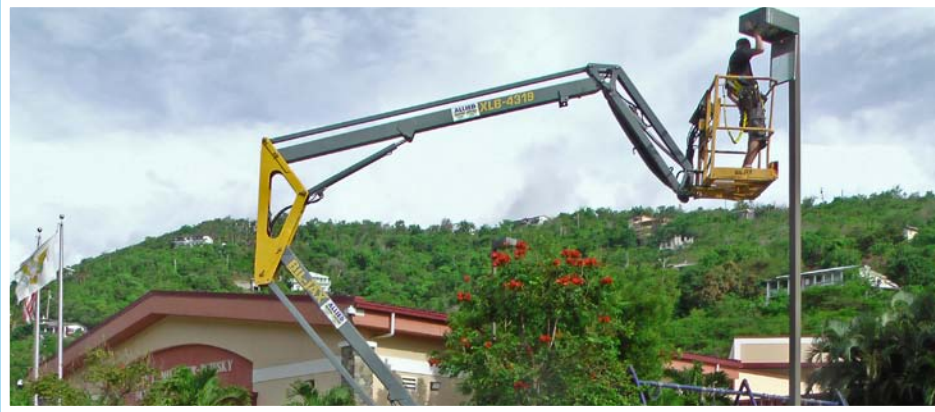
A worker installing energy-efficient outdoor lights at Yvonne E. Milliner-Bowsky Elementary School on St. Thomas. Photo from Don Buchanan, VI Energy Office
