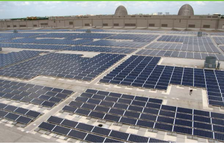
The solar array rooftop system on the south concourse of the Orange County Convention Center was completed in 2008 as a DOE Solar America Showcase. Photo from Orange County Convention Center, NREL/PIX 18077
