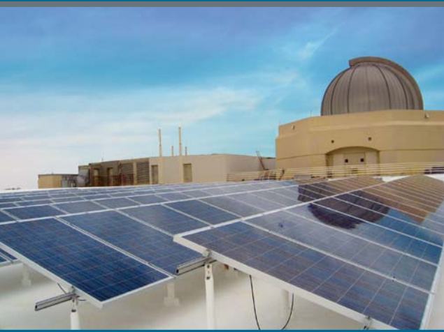
The Orlando Science Center features rooftop PV panels. Photo from Orlando Utilities Commission (OUC), NREL/PIX18715
