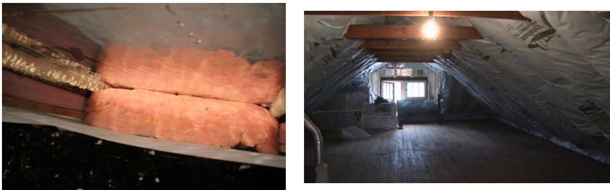
Figure 26. High density fiberglass batt in extended rafter cavity; Right: Completed roof rafter strategy (Photo credit: S. Marchese, printed with permission)
