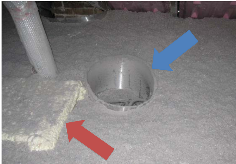
Figure 10. Bath fan housing cover encased in foam sealant (red arrow) and electrical junction box surrounded by metal insulation dam (blue arrow)
