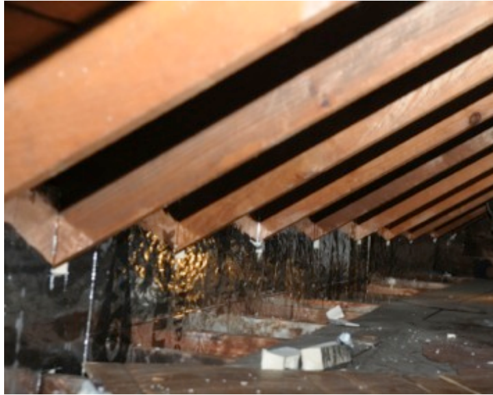
Figure 19. Foil-faced polyisocyanurate insulation notched around roof and ceiling framing (Photo credit: E. Haber, printed with permission)
