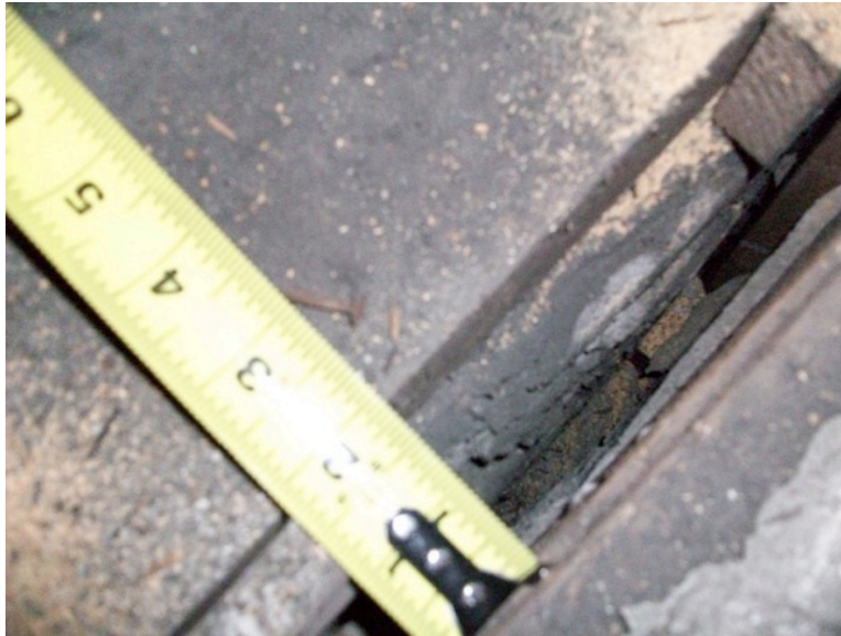
Figure 2. Furring cavity between brick masonry and interior finish as seen from the attic
