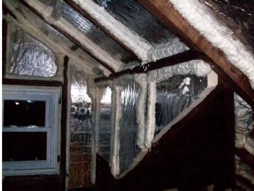
Figure 24. Foam sealant applied to seal foil-faced polyisocyanurate to surrounding framing. In this image the application of rigid insulation and foam sealant is not complete. (Photo credit: E. Haber, printed with permission)
