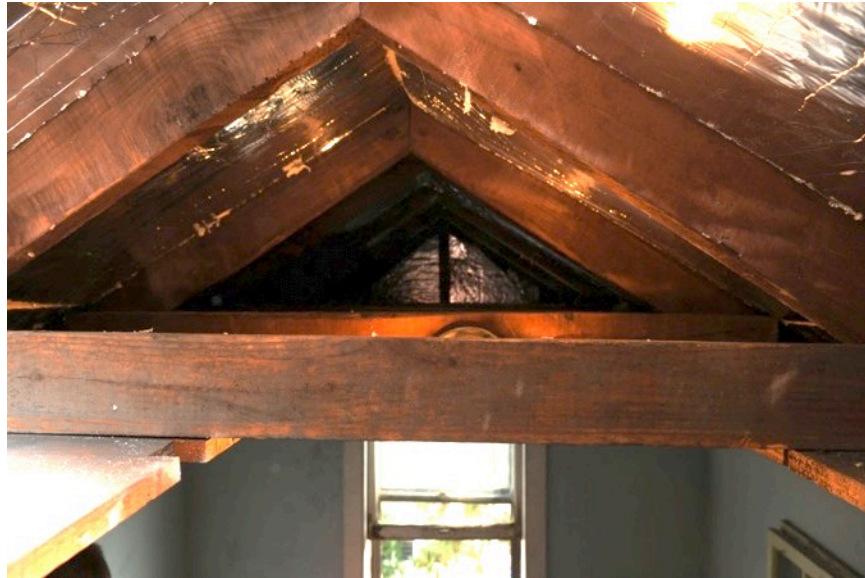
Figure 22. Foil-faced polyisocyanurate insulation installed above ceiling of finished room in attic (Photo credit: E. Haber, printed with permission)
