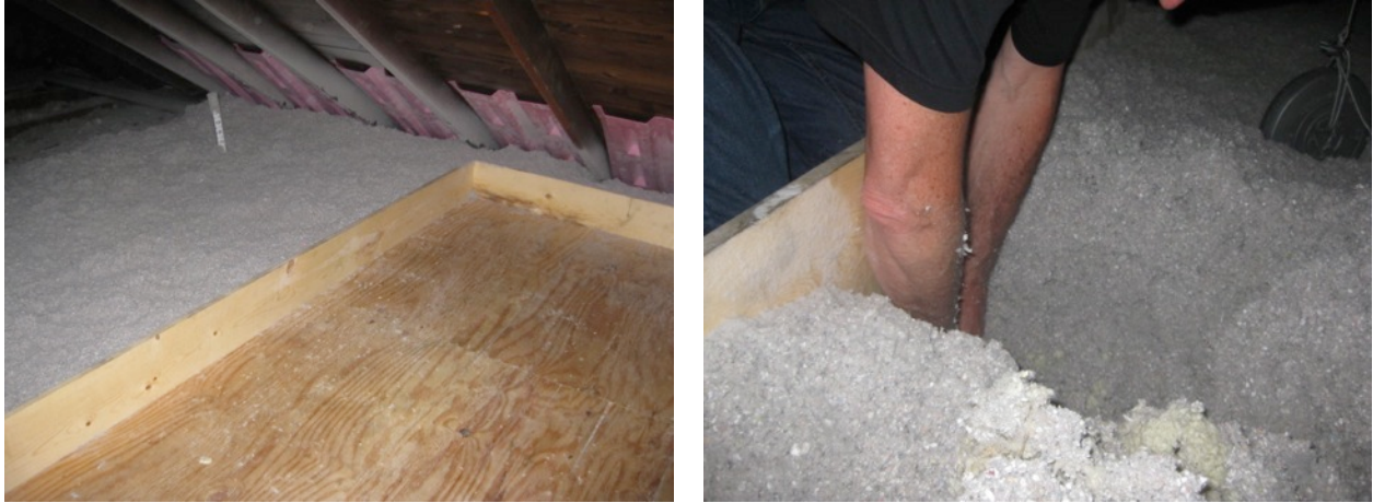
Figure 16. Left: Attic storage platform with insulation dams at the perimeter; Right: A CEDA Weatherization team member checks the depth of insulation beneath platform
