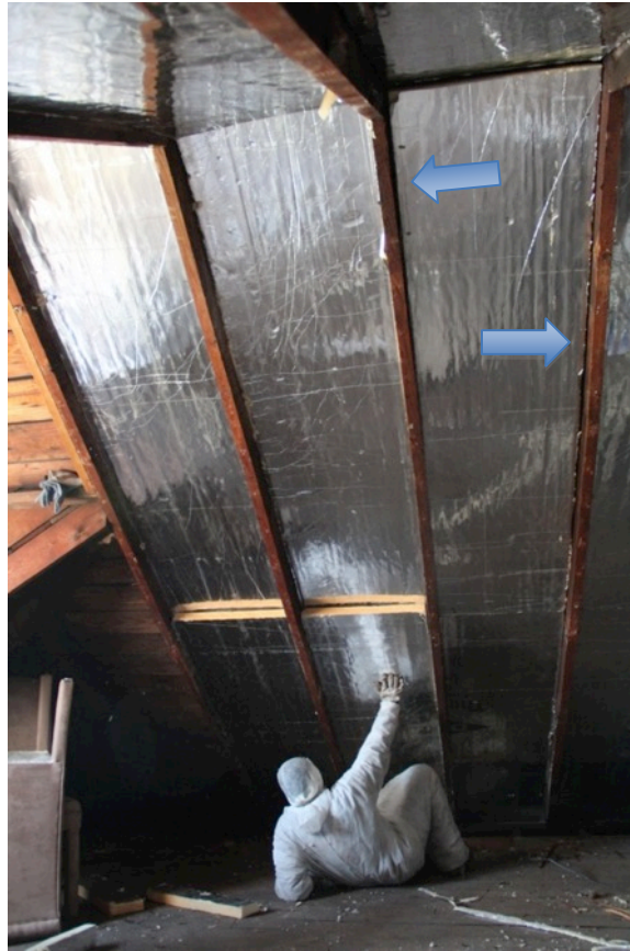
Figure 23. Foil-faced polyisocyanurate insulation fit into rafter framing cavities (Photo credit: S. Marchese, printed with permission)
