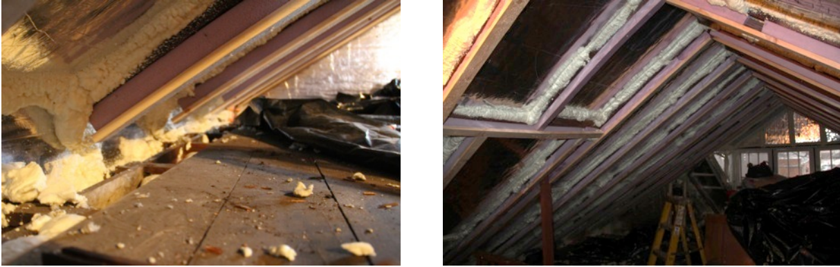
Figure 25. Left: Extruded polystyrene and wood furring strip used to extend rafter cavity; Right: Attic with rafter cavities extended in preparation for mineral fiber insulation (Photo credit: S. Marchese, printed with permission)
