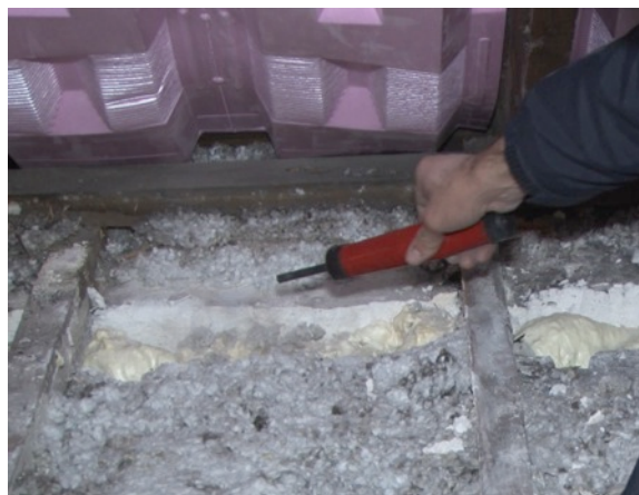
Figure 12. CEDA Weatherization assessing effectiveness of air seal at furring cavity between brick masonry and interior finish (Photo credit: S. Marchese, printed with permission)
