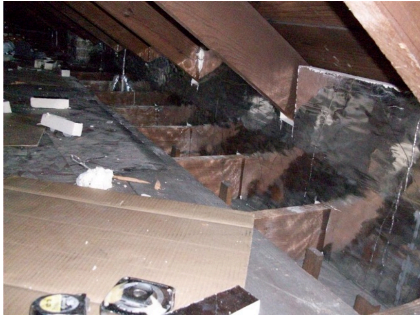
Figure 4. Foil-faced polyisocyanurate board insulation installed to transition thermal control from top of masonry wall to roof. The rigid insulation board rests on top of a wood plate at the top of the brick wall. Note that furring cavity gap (at junction of wall plaster and ceiling plaster) is to interior side of the rigid board insulation as indicated by wood furring extending above the top of the brick wall.
