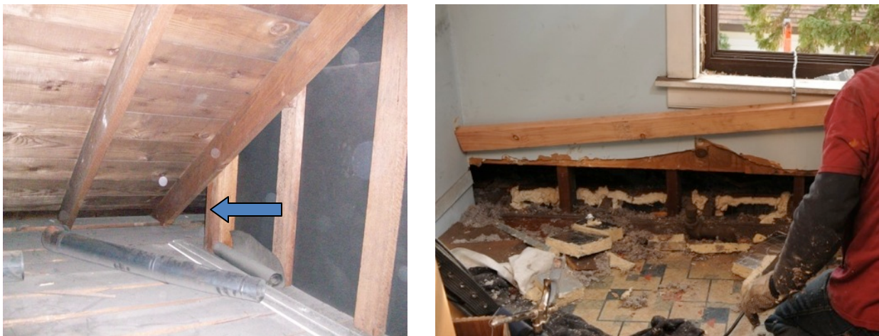
Figure 21. Left: Small space with limited access at face of dormer. Right: section of interior finish removed to allow air sealing (Photo credit: E. Haber, printed with permission)
