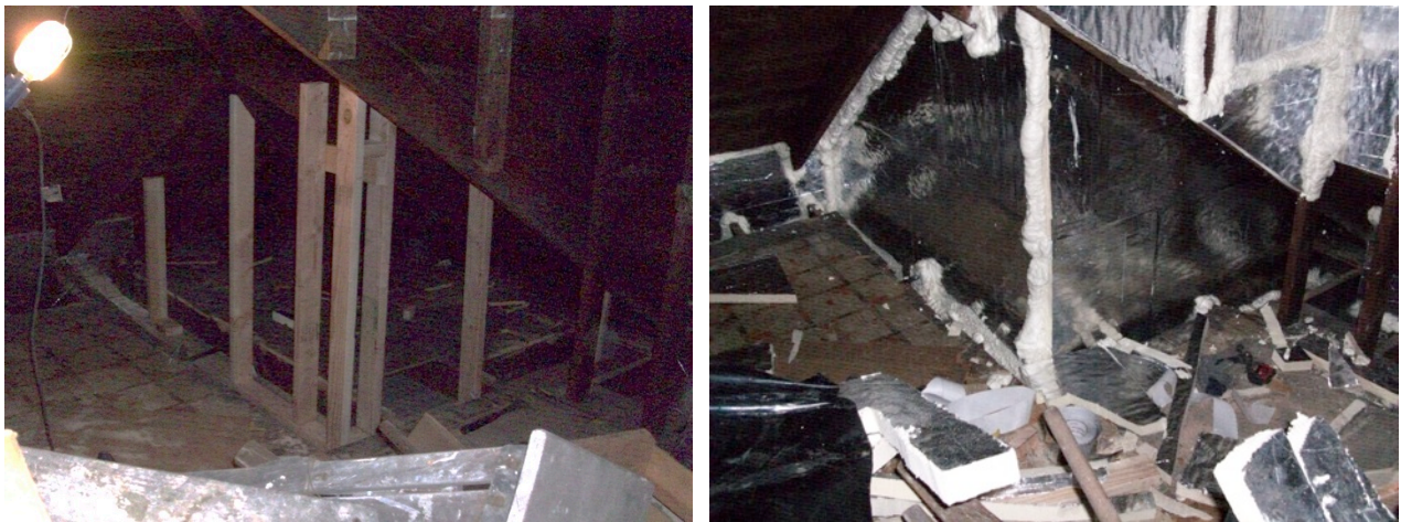
Figure 20. Left: Framing added above exterior wall at inset entry; Right: rigid board insulation installed to transition thermal control from exterior wall to roof assembly
