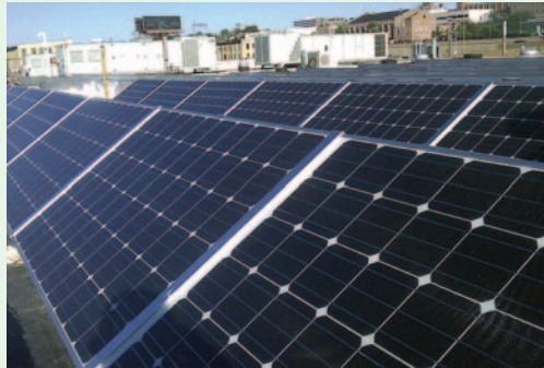
The Forest County Potawatomi Tribe's solar system is providing heating, cooling, and electricity to the Tribe's administration building in Milwaukee, Wisconsin. Photo from the Forest County Potawatomi Tribe, NREL/PIX 20107
