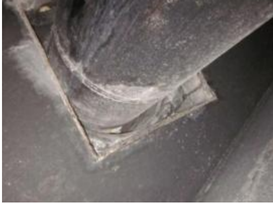
Large gap around the trash chute
