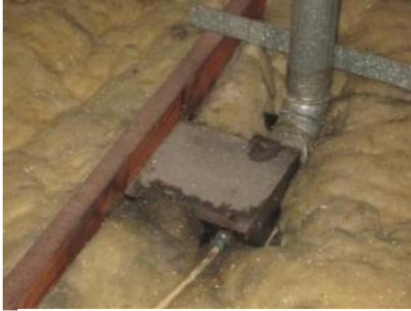
Leakage around bath fans is apparent from stained fiberglass
