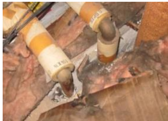
Pipe penetrations into living space
