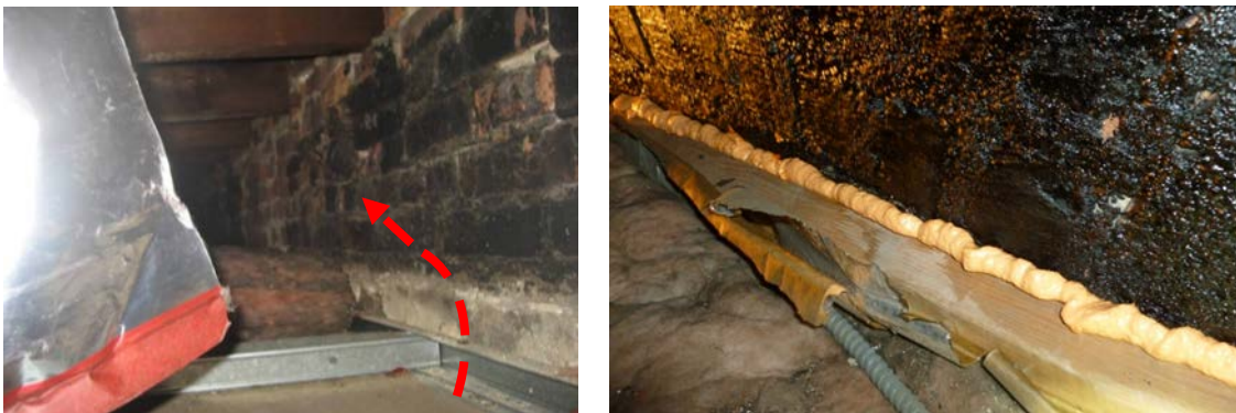
Figure 27. Typical leakage location at exterior wall and arrow showing path of air movement (left). Gap sealed using one-part expanding foam (right).
