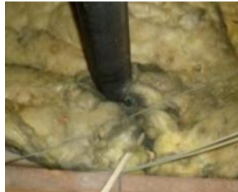
Figure 6. Dirty insulation suggests air movement. The insulation is acting as a filter
