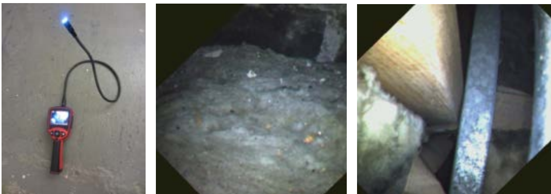
Figure 9. Remote inspection with a borescope (from left to right): Borescope tool; finding existing insulation; finding major air leaks despite past insulation work.
