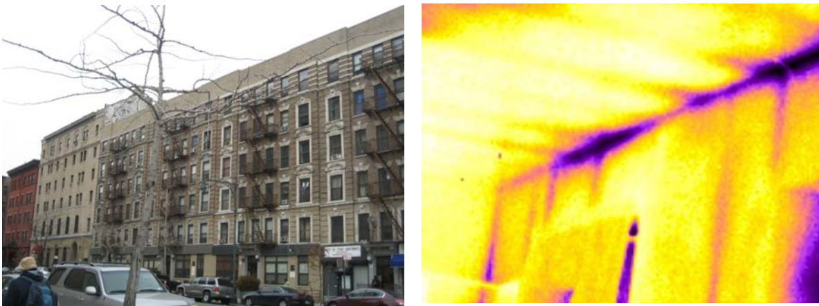
Figure 11. Using infrared imaging to detect air leaks on a cold day. The image on the right shows potential air leakage at the ceiling/wall intersection on the top floor that should be further inspected.
