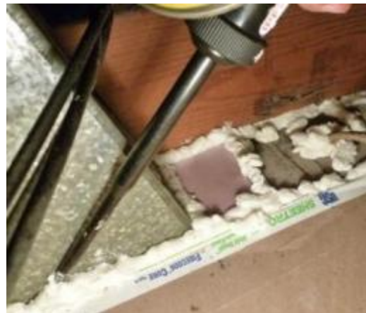
Figure 18. One-part foam effectively air seals these small irregular gaps at a duct penetration and top plate in an attic
