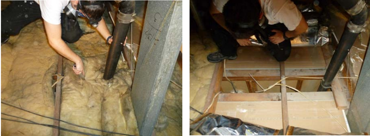
Figure 8. Without removing the attic insulation, this wall chase would have been missed
