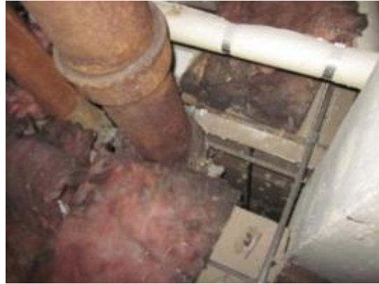
Numerous plumbing chases
