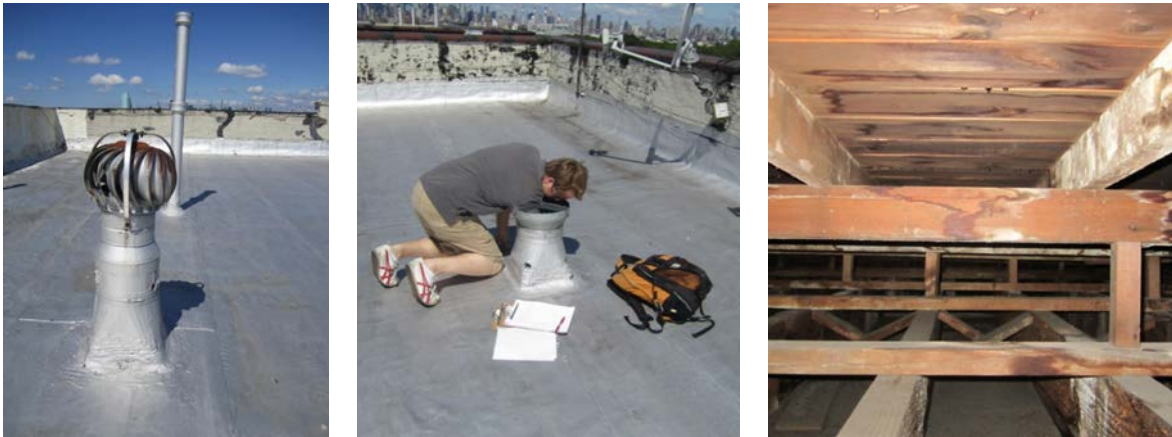
Figure 10. Using existing roof vents to investigate the roof cavity (from left to right): an existing roof vent; vent removed; view from hand-held digital camera
