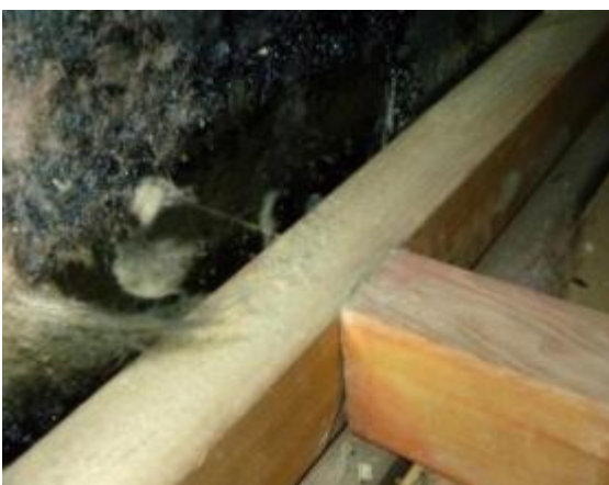
The gap between the exterior masonry wall and wall furring/ceiling must be sealed
