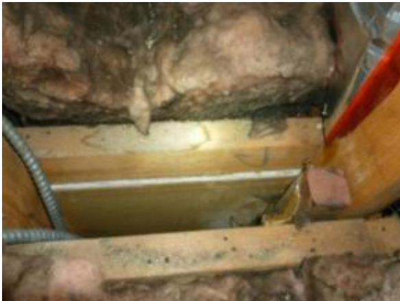
No top plates between some rooms allow air from wall cavities to escape
