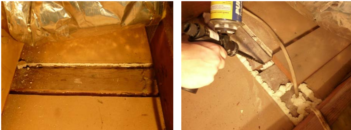
Figure 25. Common partition wall gap (left). Expanding foam quickly seals gaps at top plates (right).
