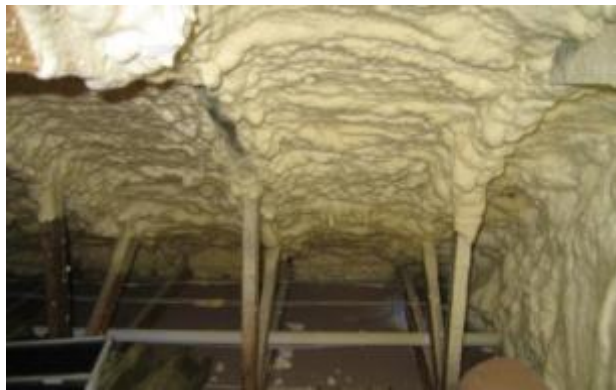
Figure 16. Polyurethane foam applied against underside of roof deck to convert to an unvented ceiling assembly
