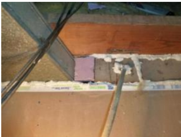
Spray foam seals smaller gaps and pieces of rigid board bridge larger gaps
