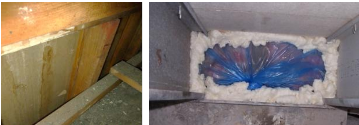
Figure 31. Open stud cavity (left) and stud cavity sealed using bagged insulation and spray foam (above).
