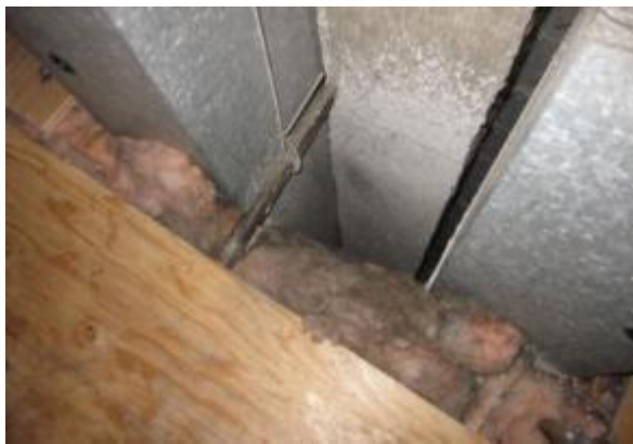
Chases around duct work
