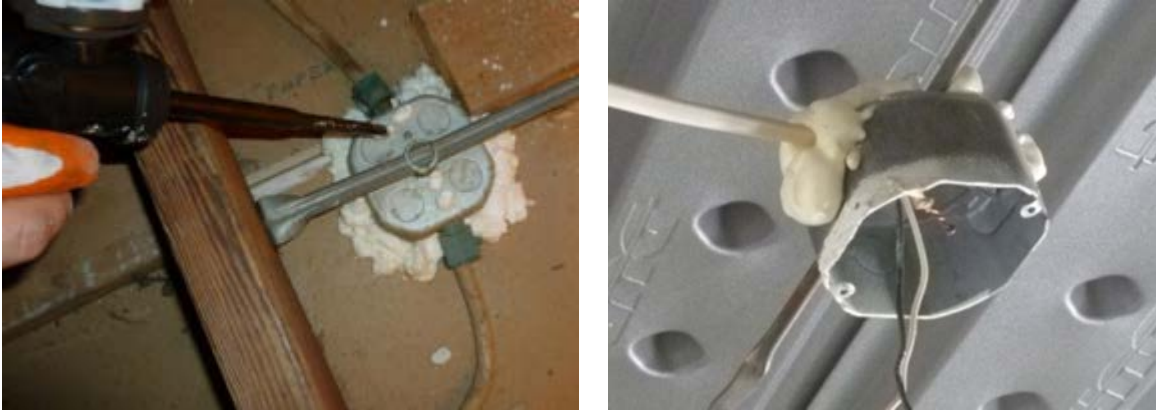
Figure 24. Sealing a common electrical penetration (left). Electrical box sealed before drywall installation (right).
