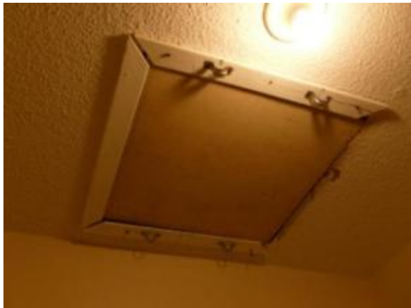
Attic hatches will receive weather-stripping and latches to hold them tightly closed
