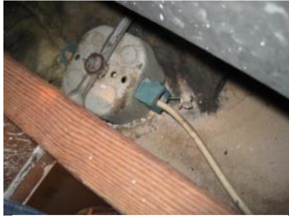
Electrical penetrations abound
