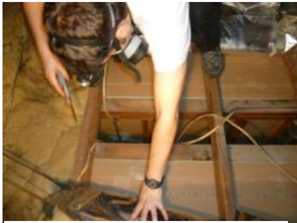
Large soffits and plumbing walls are wide open to the attic
