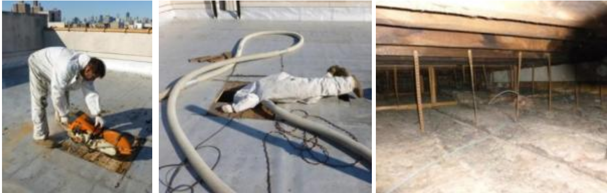
Figure 13. Accessing an attic through a cut-out in the roof (from left to right): A hole is cut with a saw; workers enter to perform air sealing; the available space in this attic affords good access.
