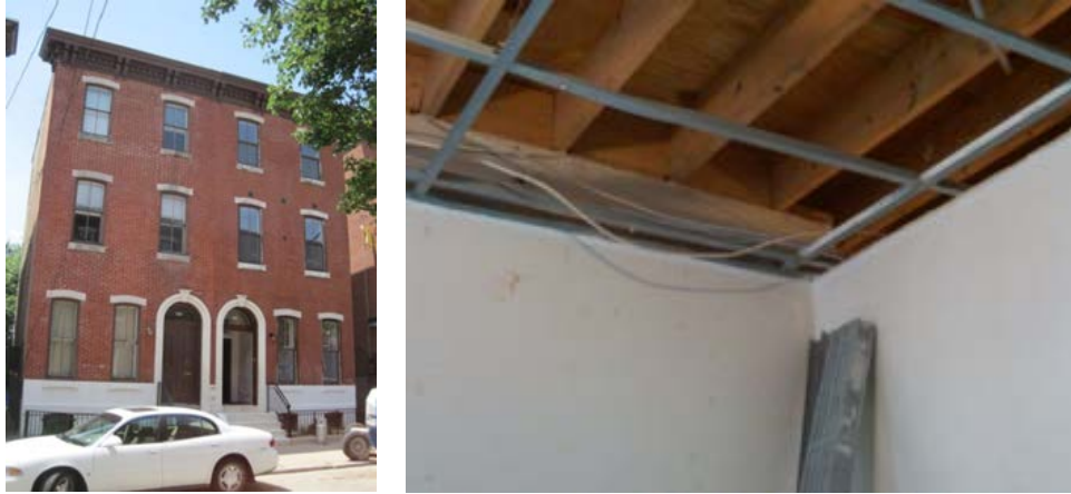
Figure 5. This multifamily building has almost no clearance for workers to enter the attic, so the only way to properly seal the cavity is from below by removing the ceiling
