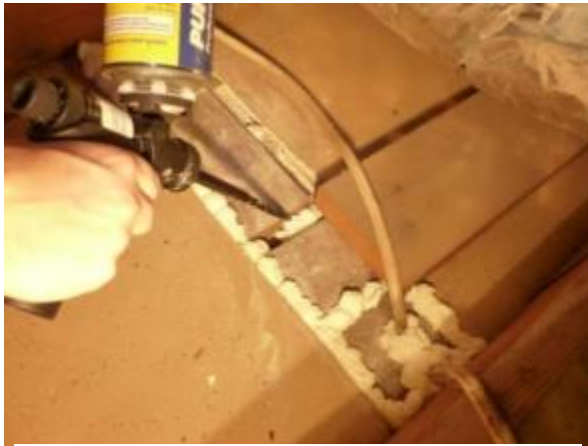
Top plates between rooms allow air from wall cavities to escape
