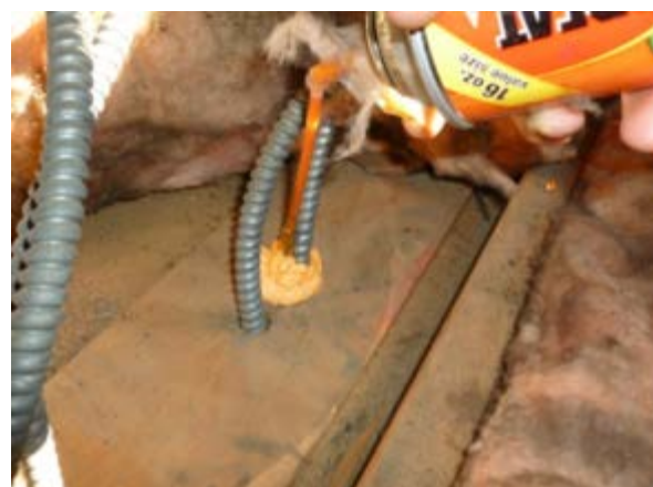
Numerous electrical penetrations contribute to leakage
