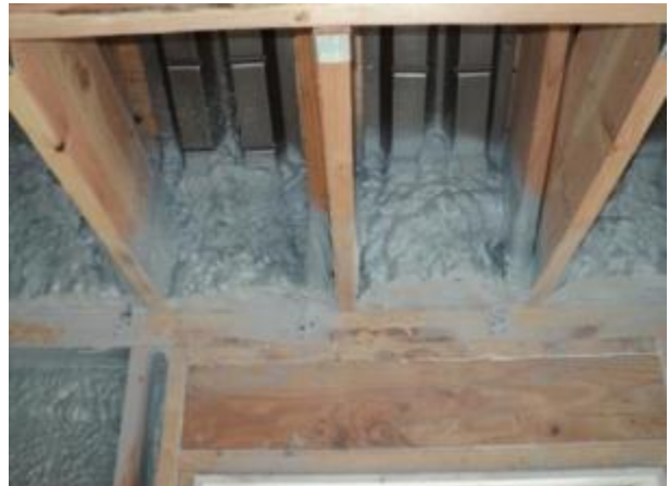
Figure 17. Closed-cell spray polyurethane foam quickly air seals and insulates this roof/wall/ceiling intersection
