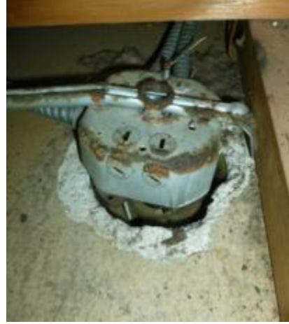
Junction boxes for lights can be quite leaky
