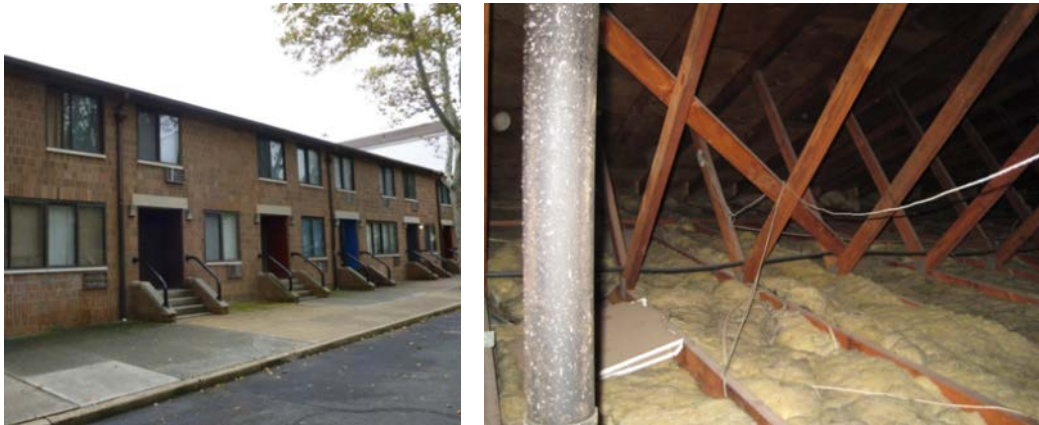
Figure 3. This complex of row houses has attics with excellent access for air sealing, as roof trusses provide plenty of maneuvering space
