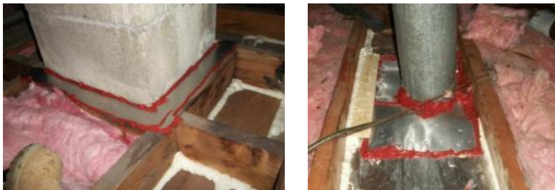
Figure 34. Sheetmetal blocking around chimneys Insulation dams still need to be installed. (Photos courtesy of Next Step Living, printed with permission)
