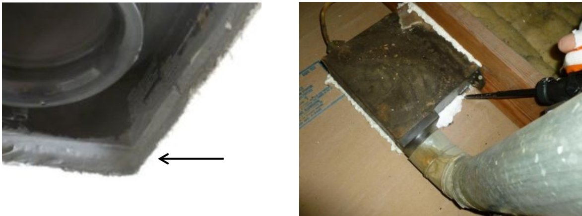
Figure 38. Caulked gap at apartment side of fan penetration (left). Sealing bath fan penetration with foam from attic side (right).
