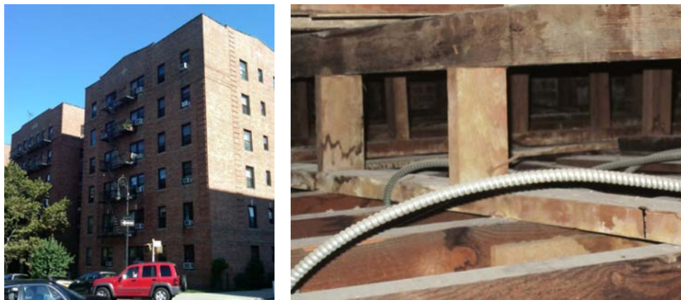
Figure 4. Access to the attic in this multifamily building will be more difficult but not impossible
