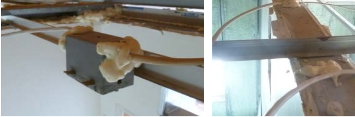
Figure 15. Air sealing junction boxes and top plate penetrations, before ceiling drywall is installed
