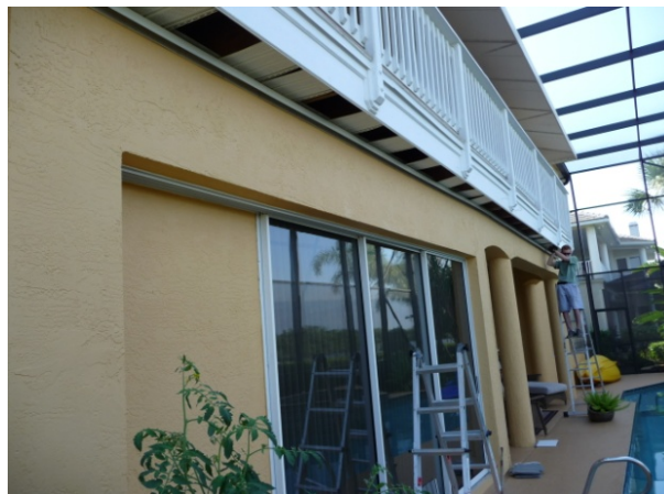
Figure 28. Soffit vent panels removed for inspection and access to seal air pathways from eave into floor cavity.
