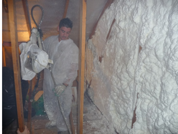
Figure 25. View of kneewall and floor cavity after being sealed with low density expansive foam.
