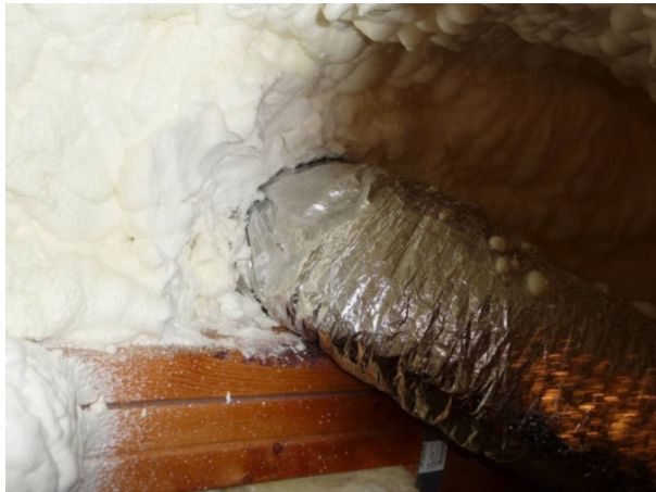
Figure 43. Supply duct from attic into floor cavity has insulation wrapped around duct before blown foam is applied.
