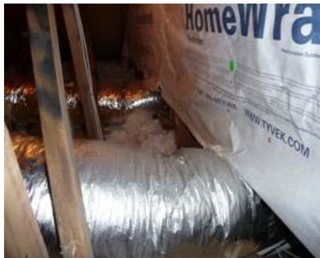
Figure 11. Flex ducts going from an attic space into the interstitial floor cavity under a portion of the second story conditioned space.
