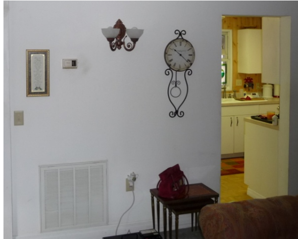
Figure 61. The interior of a return plenum, located under an AHU, can be accessed through the return grille for inspection.
