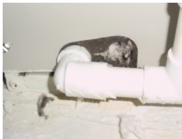
Figure 47. Loose-fill insulation has been sucked into condensate drain penetration leak.
