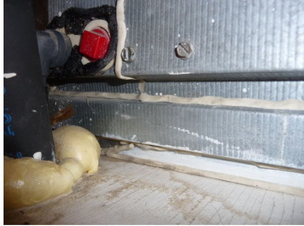
Figure 50. Black cork tape applied around condensate line penetrations and rope putty applied over seams. Expanding foam seals refrigerant line penetration into return support plenum.
