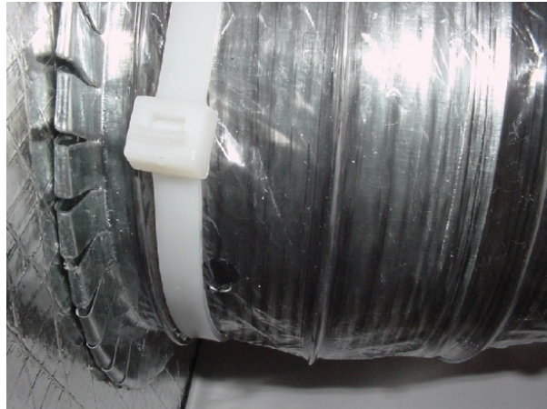
Figure 63. To make this repair, pull back the outer insulation jacket of the flex duct to expose the inner duct connection. Remove the strap and inner duct from metal collar. Remove any loose tape.
