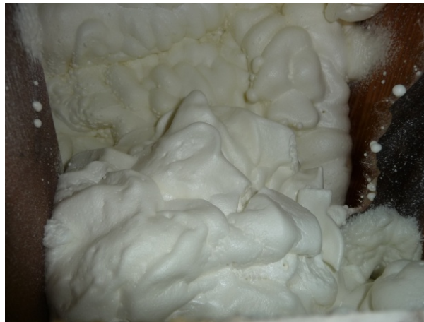
Figure 39. The next step is to complete the seal from floor deck vertically down to the bottom of the soffit surface. This is done between each joist section.
