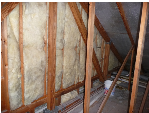
Figure 21. View of kneewall and portions of open floor cavity as seen from inside the attic.
