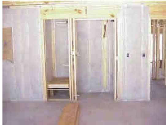
Figure 16. An insulated garage closet located will house an AHU. A weather stripped door will isolate the closet from the garage. A vent from the closet to indoors would also further enhance the system operating efficiency.
