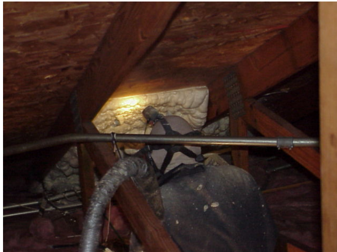
Figure 44. To encapsulate the attic space, spray foam is applied to vents and roof deck. Foam application starts low, at the top of exterior wall, sealing off the vented eave from the attic then continues to completely cover the entire roof deck.
