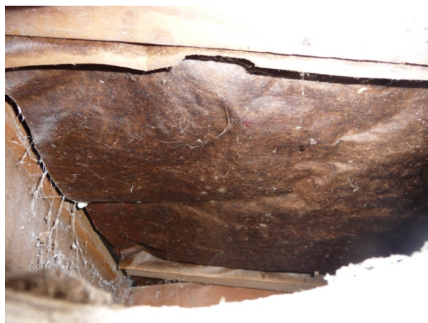
Figure 37. Insulation batts were present in most of the eave areas providing some thermal protection for the floor above. However, because the batts did not fit tightly between the joists, they allow airflow to move into the floor cavity.
