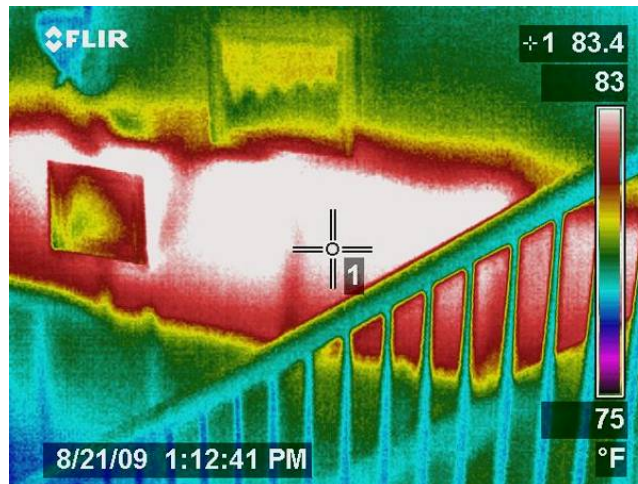
Figure 13. Infrared image of stairwell showing elevated wall temperature from hot air in an interstitial floor cavity. Note location of pictures and light fixture.
