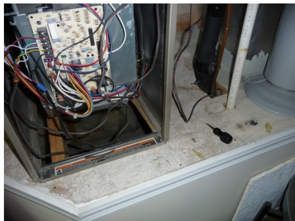
Figure 54. Front panel of furnace is removed for inspection inside the return plenum. Because of limited plenum access, part of the drywall has to be removed to provide access for plenum sealing.
