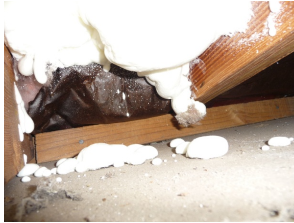
Figure 38. First, the foam spray gun is inserted into the soffit vent hole to apply foam insulation to the floor deck above, beyond the top of the exterior wall.
