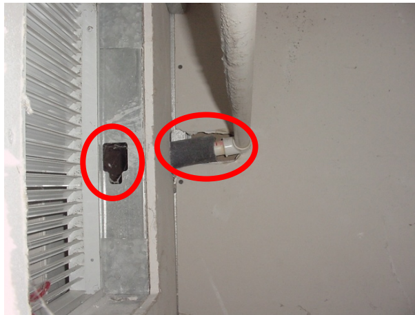
Figure 62. Grille transfer through a wall has leakage into wall cavities that need to be sealed.
