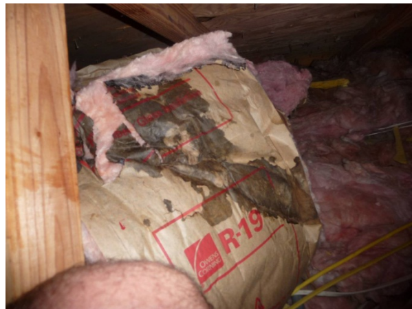
Figure 41. Batt pulled away from duct shows it is soaked where dark areas are seen on paper facing.
