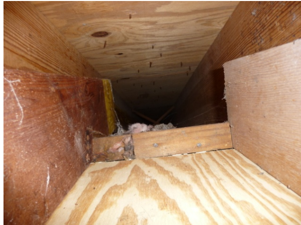
Figure 36. Connection from vented eave to floor cavity where no insulation was found.
