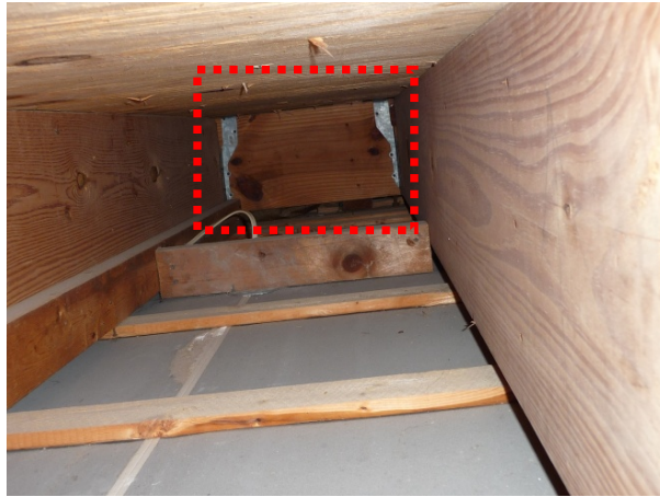
Figure 30. View from eave toward floor cavity shows pathway to floor under joist braced at back, which would be the ideal place for the air and thermal barrier in this construction.
