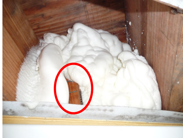
Figure 33. Spray foam expands considerably and conforms effectively around the end of a floor truss section within a floor joist.
