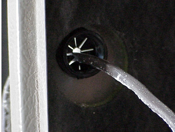
Figure 48. Leaky thermostat wire penetration.
