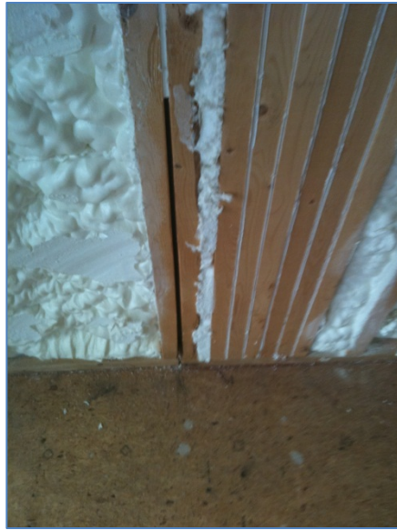
Figure 3. Over-designed framing at panel juncture
