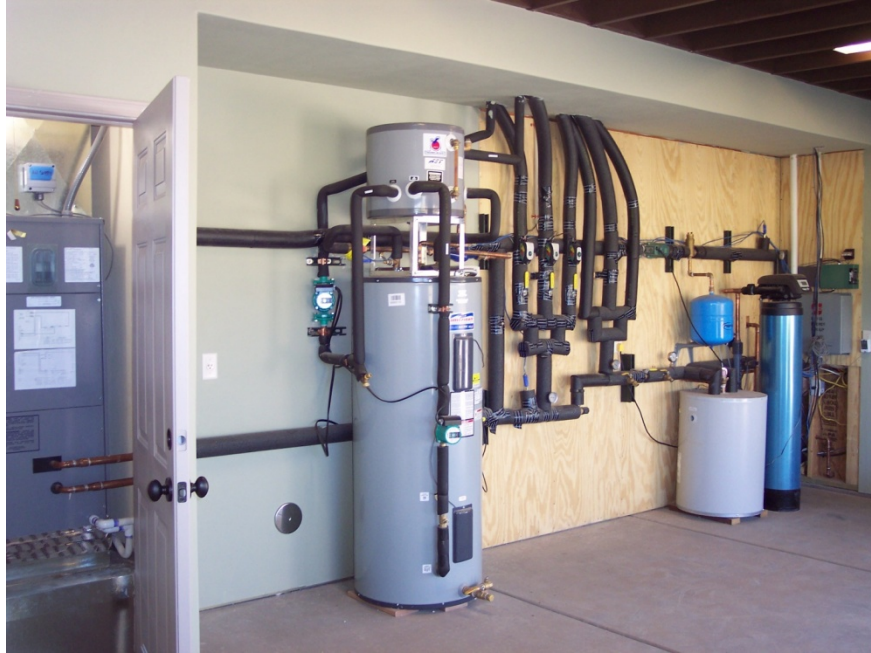
Figure 6. Hydronic equipment and piping installed in the garage
