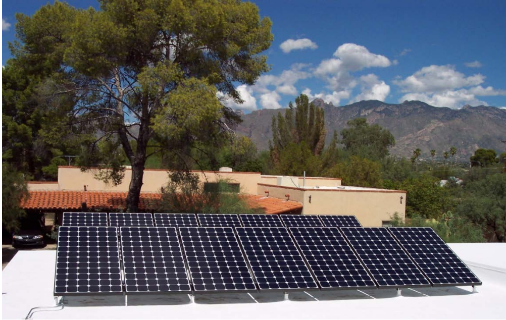
Figure 7. The 3kW photovoltaic system
