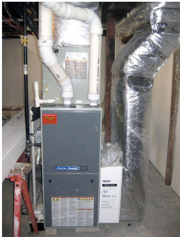
Figure 9. Belmont Two-Family natural gas furnace in basement with air-conditioner coil attached
