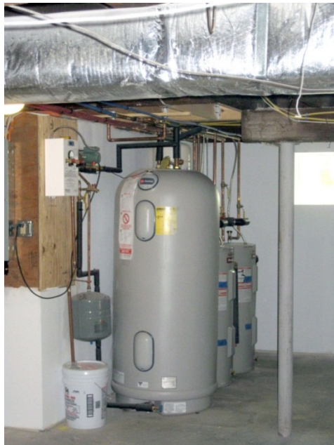
Figure 11. Belmont Two-Family DHW storage tank for solar thermal with backup electric tanks
