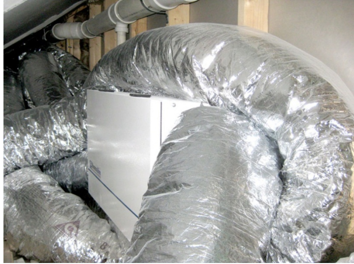
Figure 10. Belmont Two-Family ERV for upper unit in attic kneewall space
