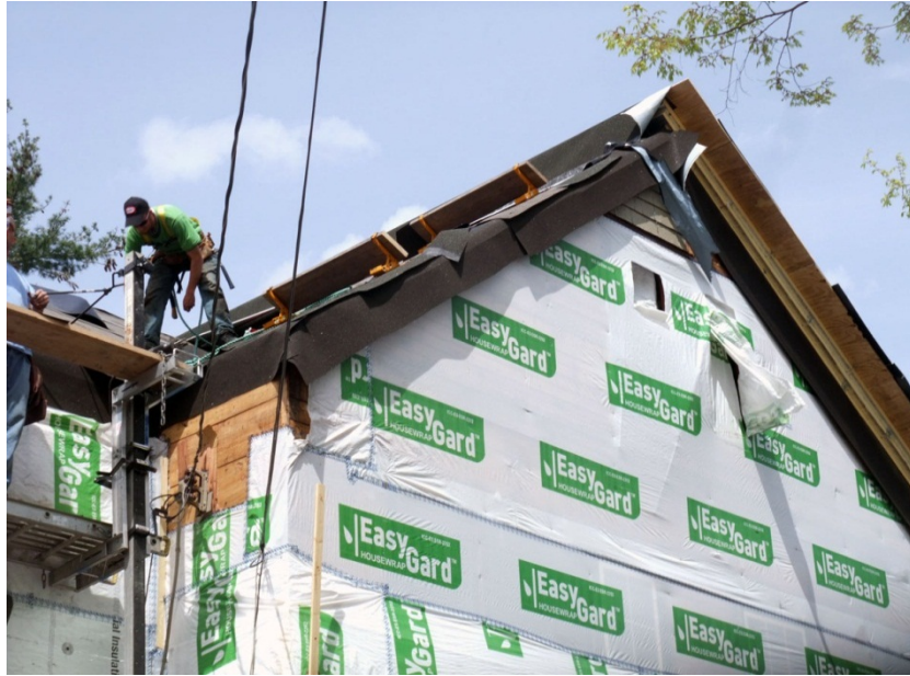
Figure 7. Belmont Two-Family, showing the roof membrane that was sealed to exterior insulating sheathing
