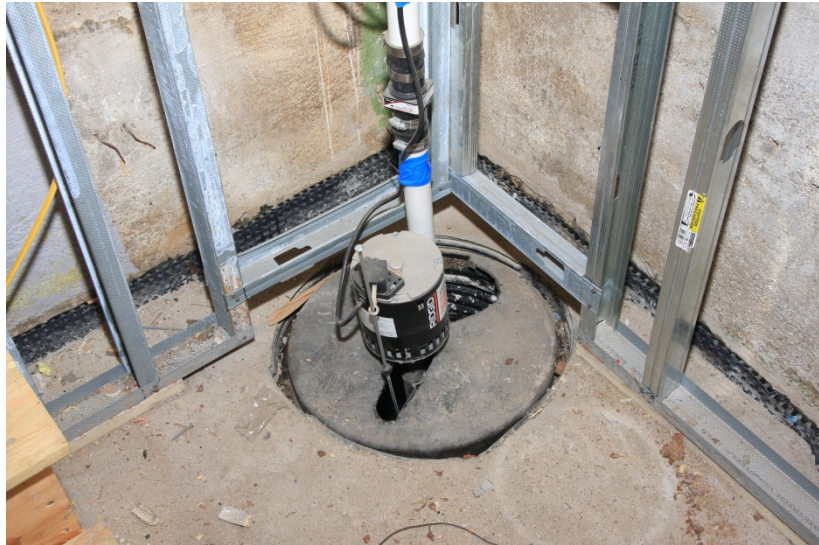
Figure 6. Belmont Two-Family sump pump installed (before basement wall was insulated)
