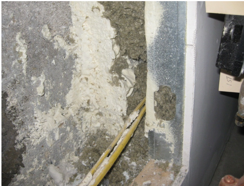
Figure 4. Belmont Two-Family basement wall insulation
