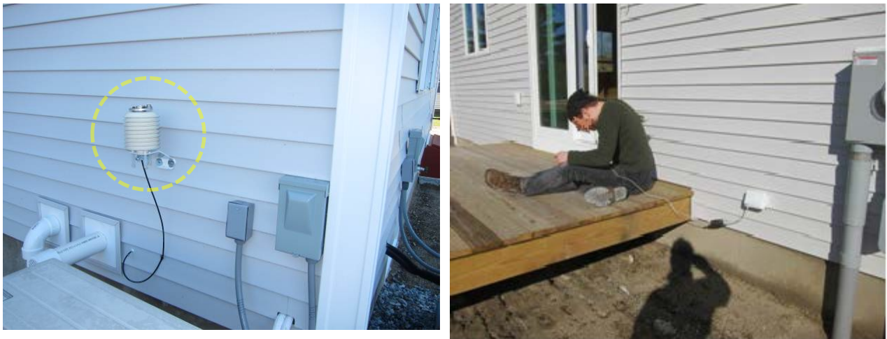
Figure 53. (L) Exterior T/RH sensor; (R) data collection from exterior connection port
