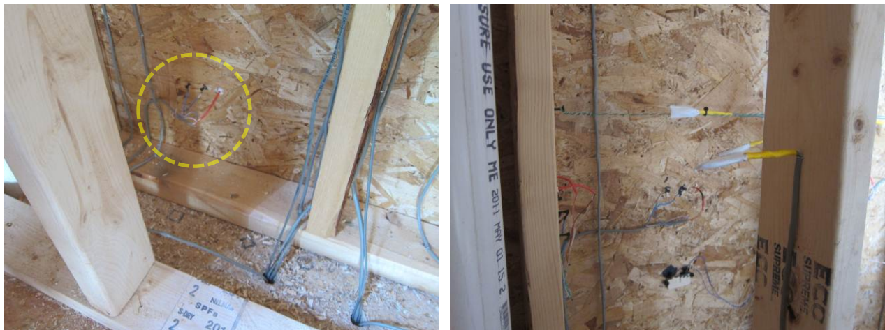
Figure 48. (L) Temperature and MC sensor at sheathing; (R) sensors at mid-height of stud bay
