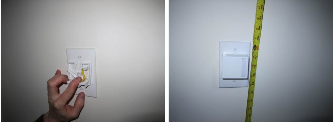
Figure 52. Sensor measure interior (bedroom) T/RH sensors
