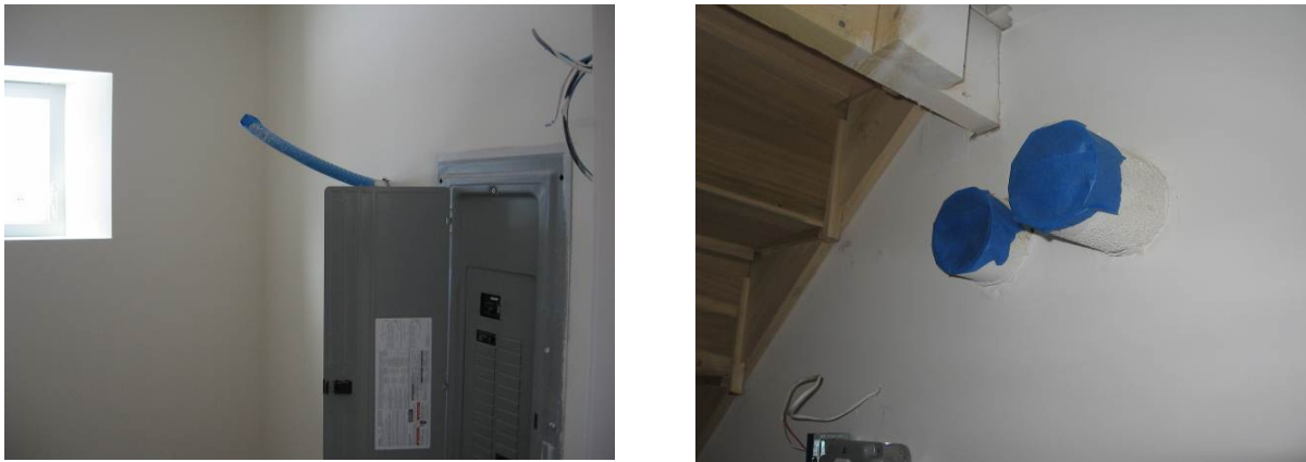
Figure 18. (L) PV inverter connection; (R) tankless water heater intake and exhaust vent
