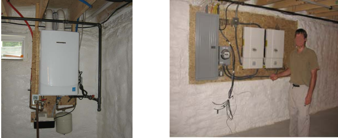
Figure 66. (L) Tankless water heater; (R) PV inverters in unfinished basement
