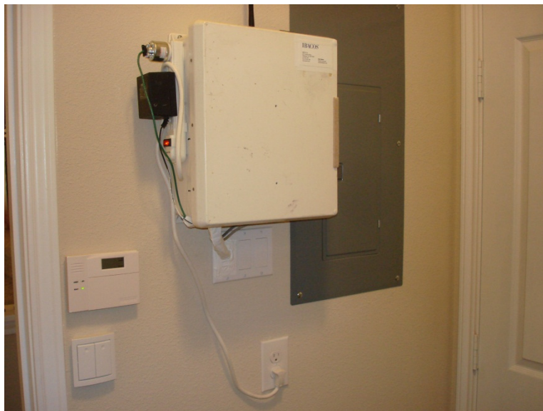
Figure 29. Location #8; wires at the data logger location near the indoor electrical panel
