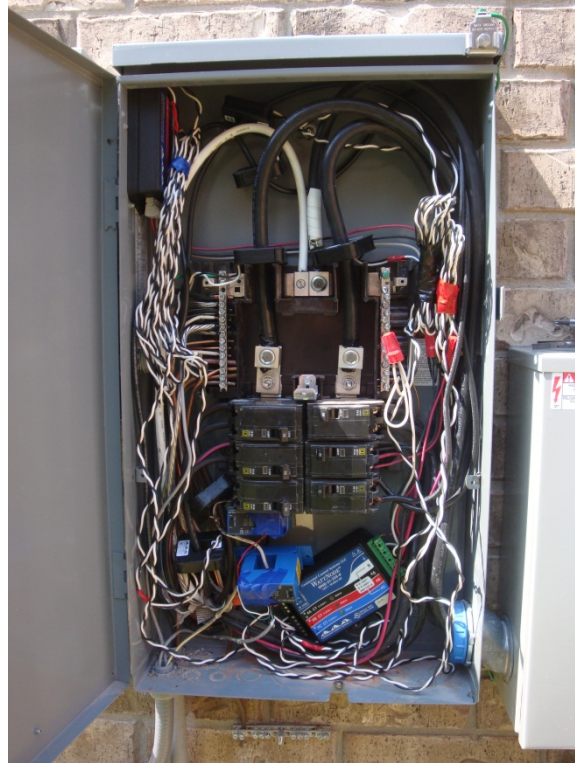
Figure 28. Location #7; electrical measurements at the outdoor electrical panel
