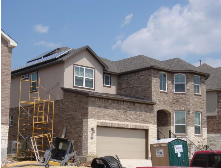
Figure 24. Location #3; incident solar radiation sensor on the roof in plane with solar DHW and PV panels
