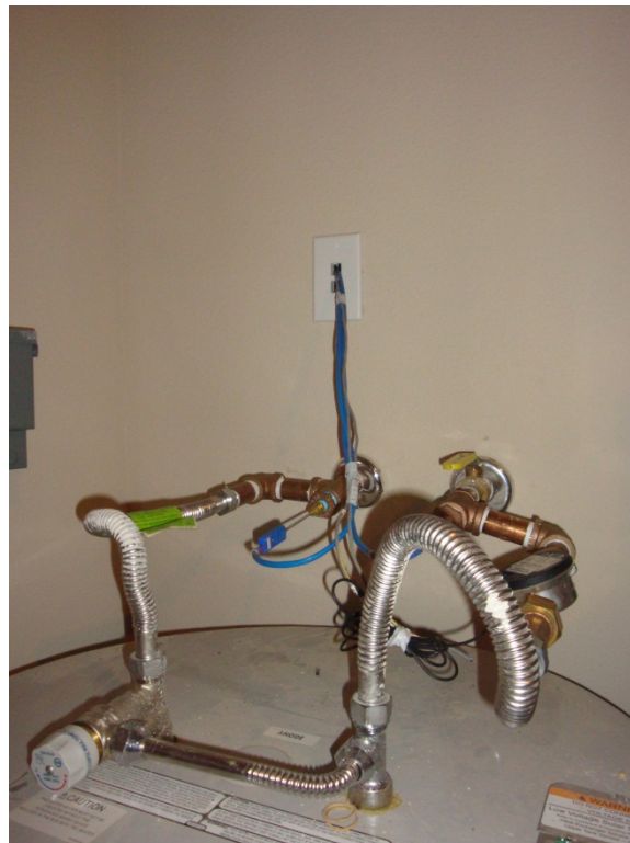
Figure 27. Location #6; flow and temperature measurements at the water heater location
