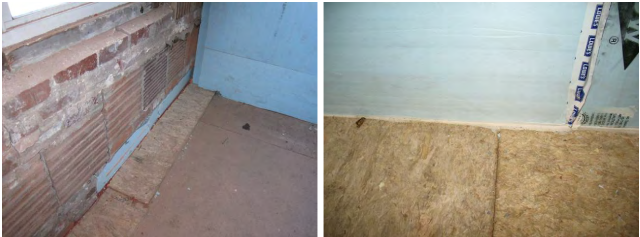
Figure 45. (L) Floor edge detail, showing added floor sheathing; (R) air seal between foam and floor
