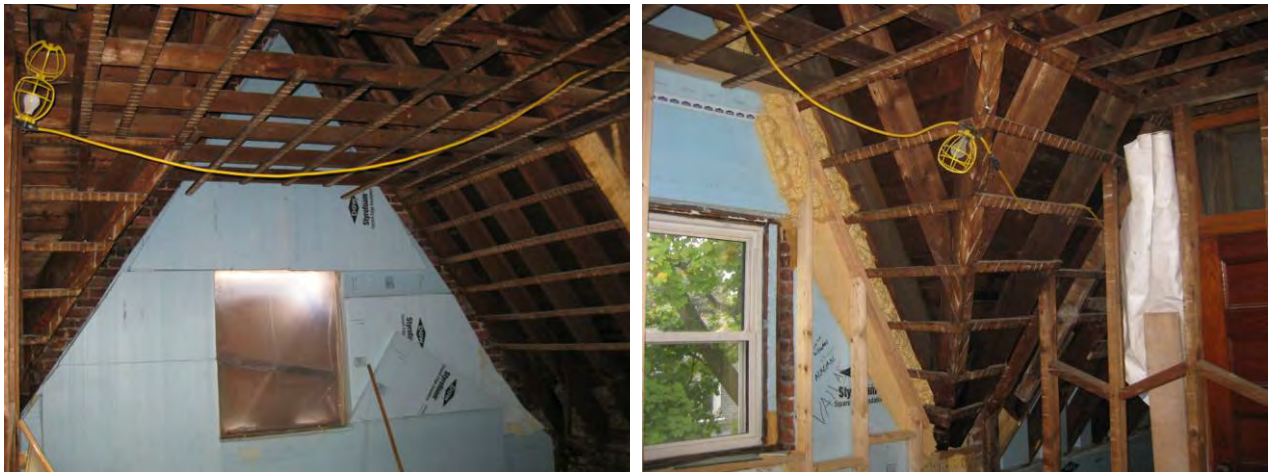
Figure 34. (L) Rigid wall insulation left clear of roof; (R) infill with spray foam kit
