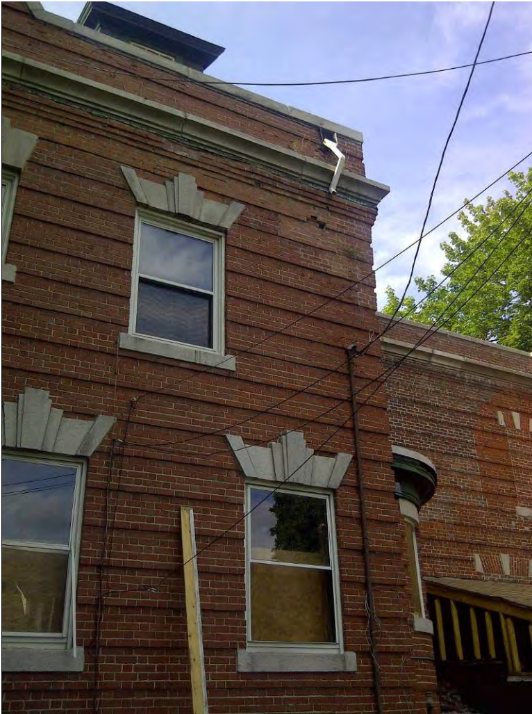
Figure 9: Original building – missing downspout
