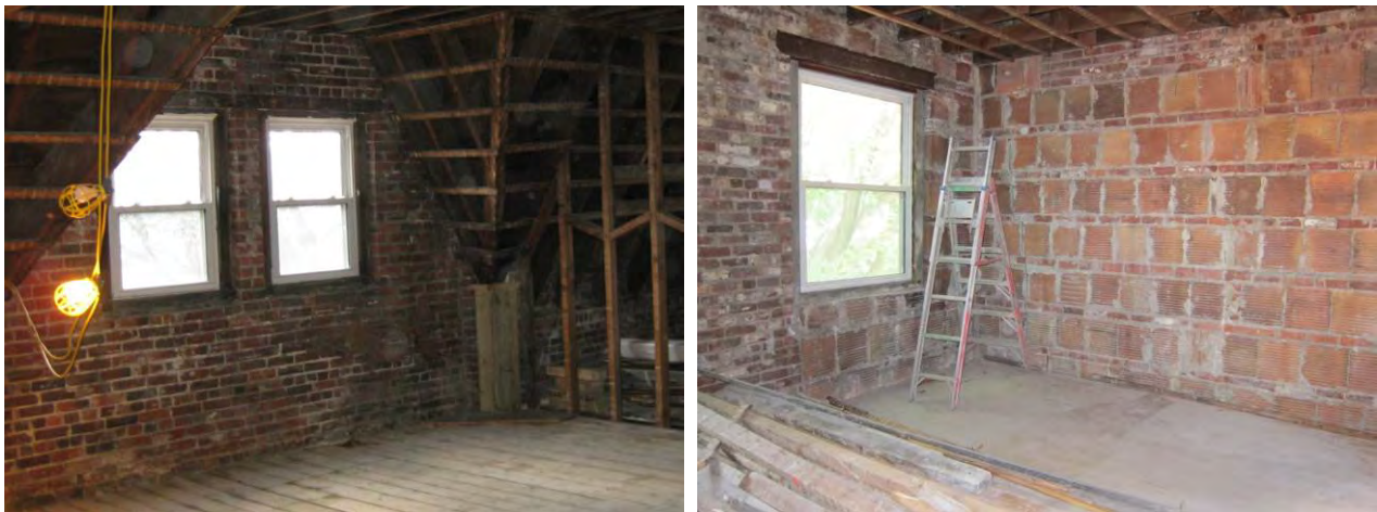
Figure 22. (L) Exterior wall conditions at solid brick; (R) hollow clay block infill conditions
