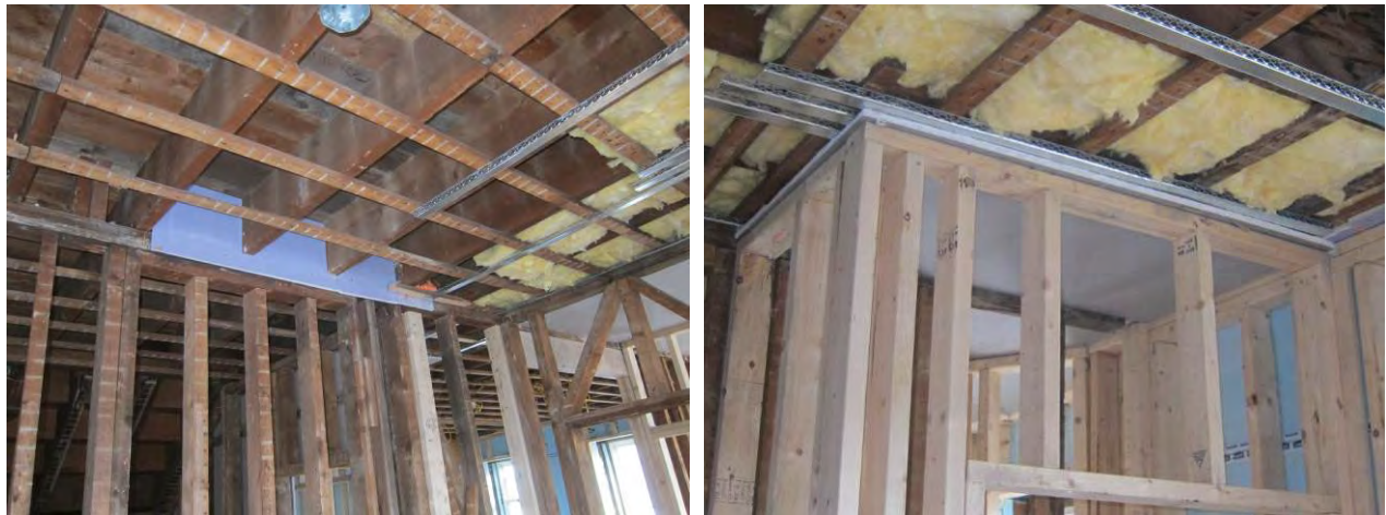
Figure 50. (L) Notched gypsum board at demising wall; (R) ceiling gypsum board continuous over unit interior partition walls
