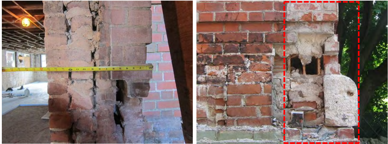
Figure 23. (L) Wall section at solid brick; (R) at hollow clay block infill conditions
