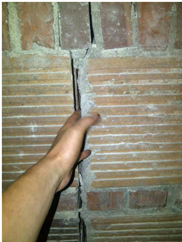
Figure 28: Addition – interior view of a crack in the masonry mass wall
