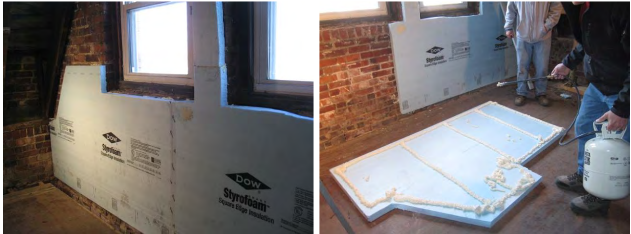
Figure 24. (L) Test installation of foam on masonry; (R) use of polyurethane adhesive
