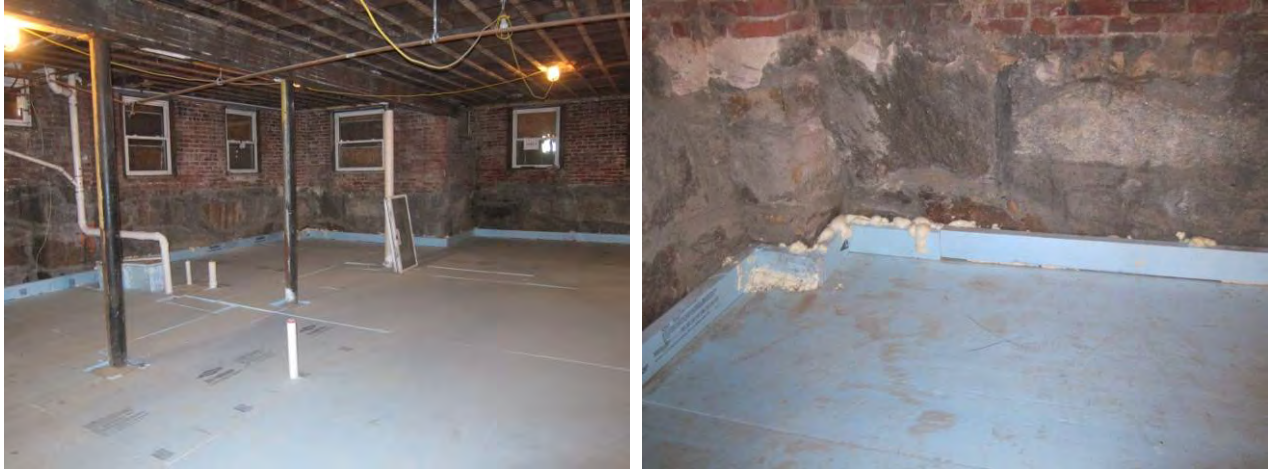
Figure 39. (L) Installed subslab insulation at basement; (R) detail of slab edge insulation
