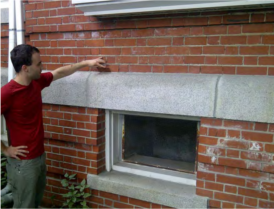
Figure 7: Original building: brickwork spalling and surface efflorescence
