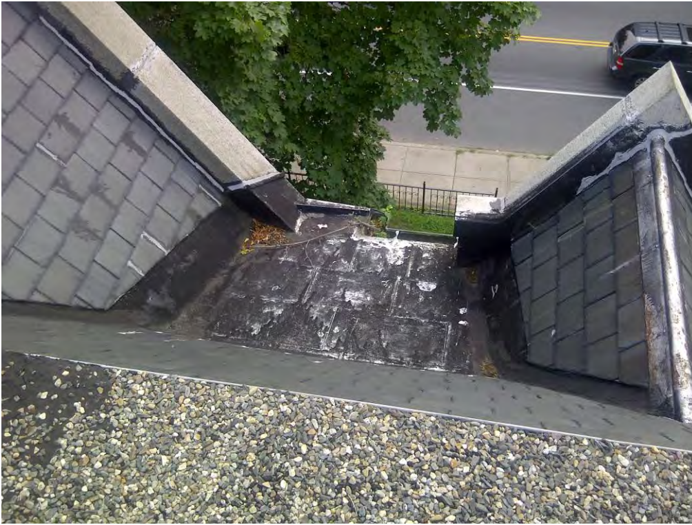
Figure 12: Roof drain filled with debris
