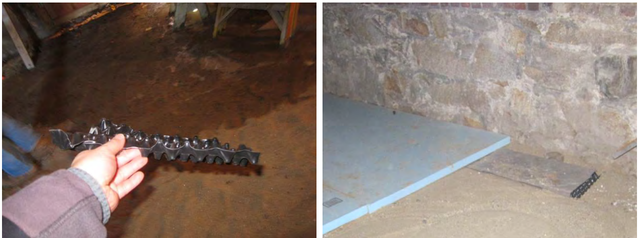
Figure 38. (L) Dimpled core of radon vent mat; (R) radon vent map installed under XPS
