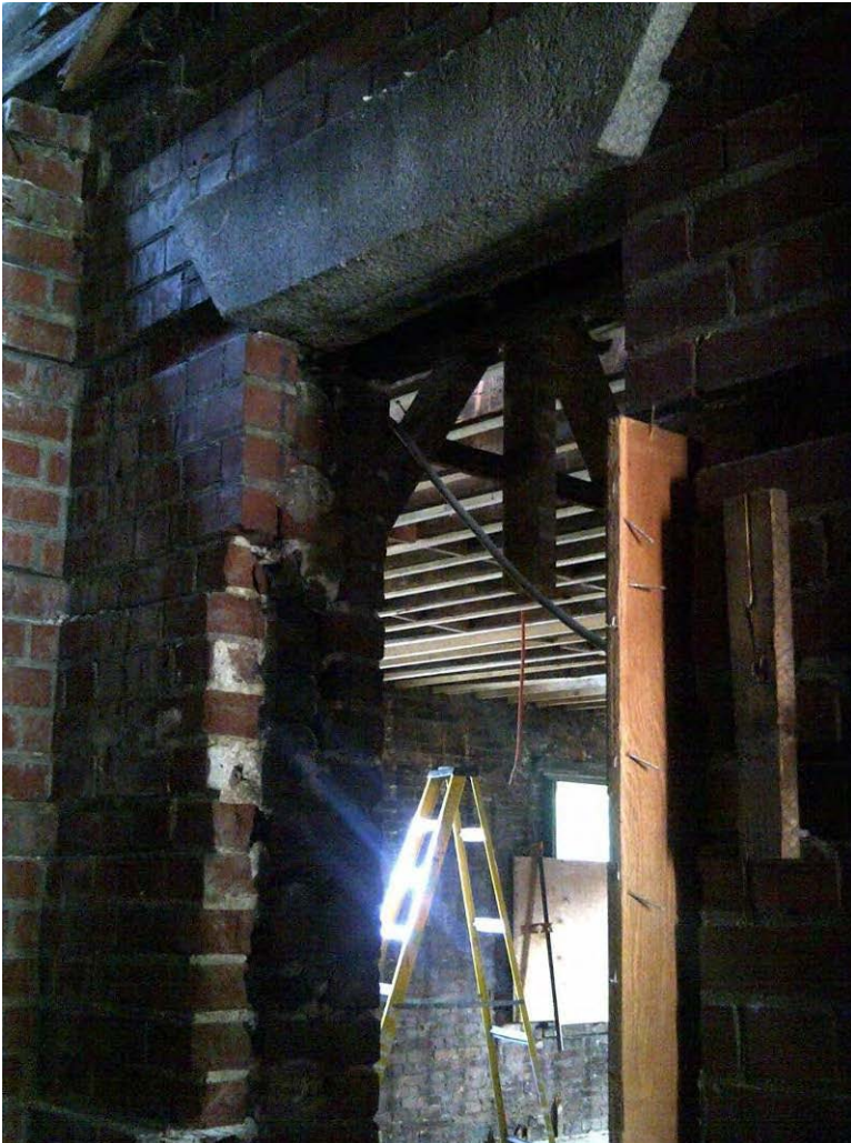
Figure 2: Original building – view of masonry wall section where doorway was shifted to interior
