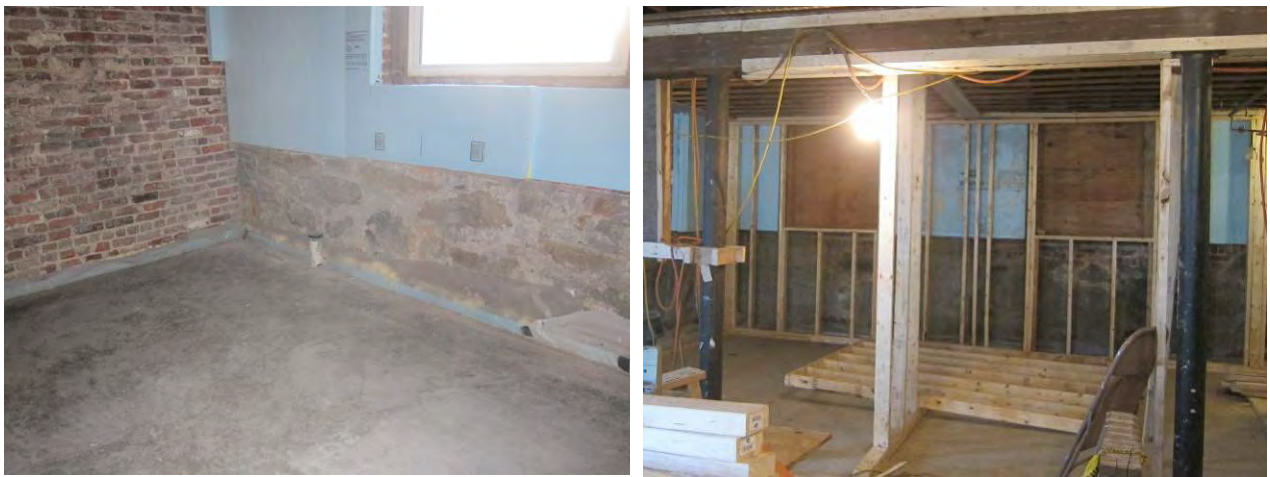
Figure 40. (L) Edge detail after casting of slab; (R) installation of interior framing
