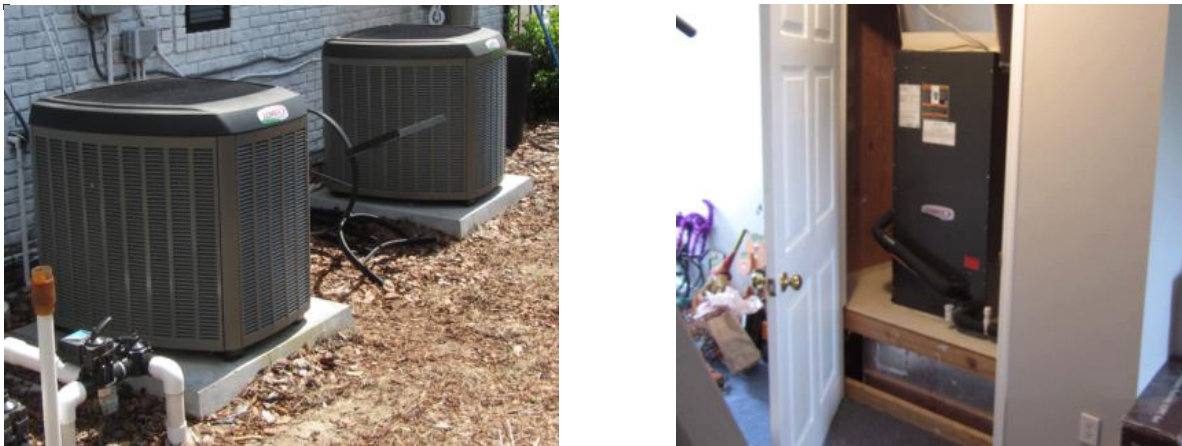
Figure 7. Outdoor condensers and the AHUs for the second floor
