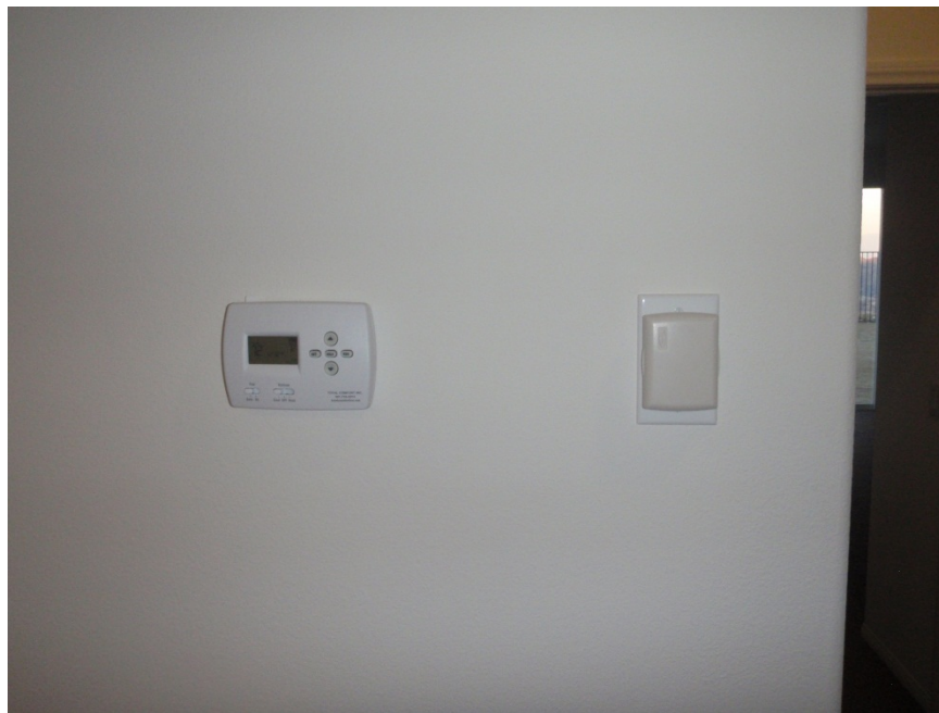
Figure 4. Temperature and RH sensor at the thermostat location
