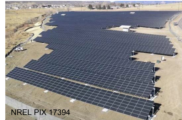
Ft. Carson 2MW Solar Array
