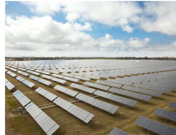
Photo by SunPower Corporation, NREL 23816
