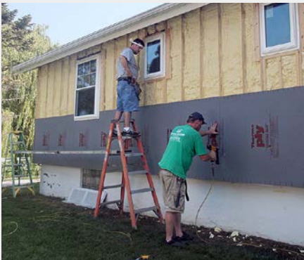
The framing is in place, spray foam is installed, and T-Ply is being installed. The next step is new siding.
