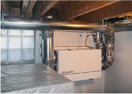
The team also installed a new energy recovery ventilator in the basement and used spray foam to insulate the rim band joists.
