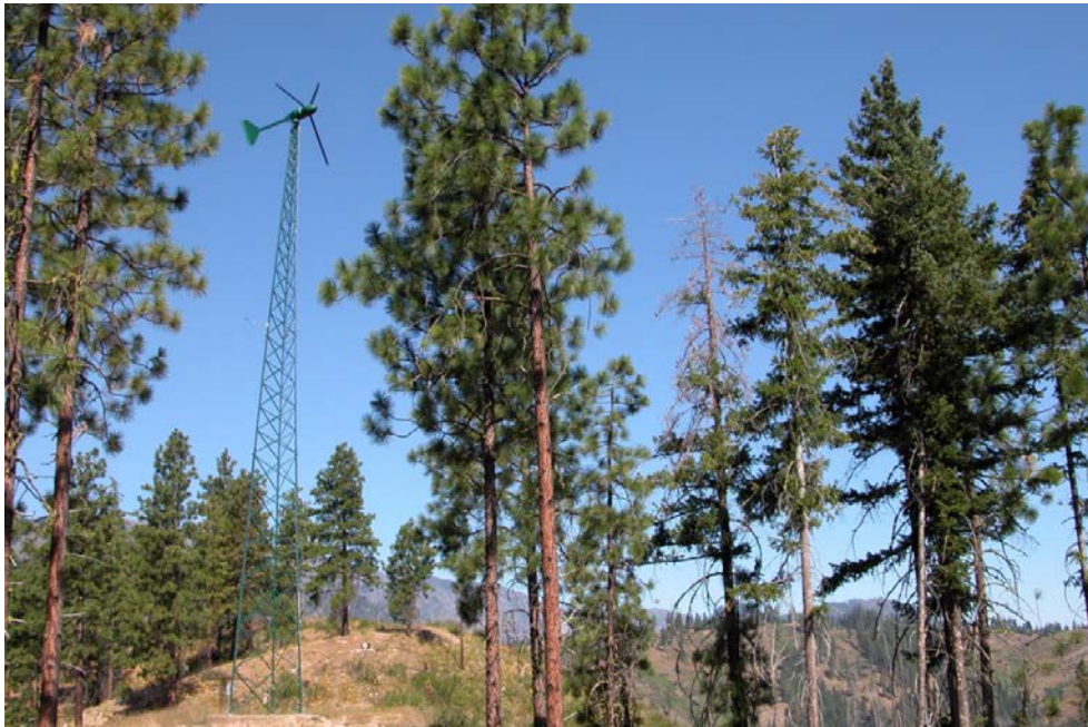
Bergey Excel 10, 10-kW turbine; Peshastin, Washington, Photo by Abigail Krich, NREL 13495
