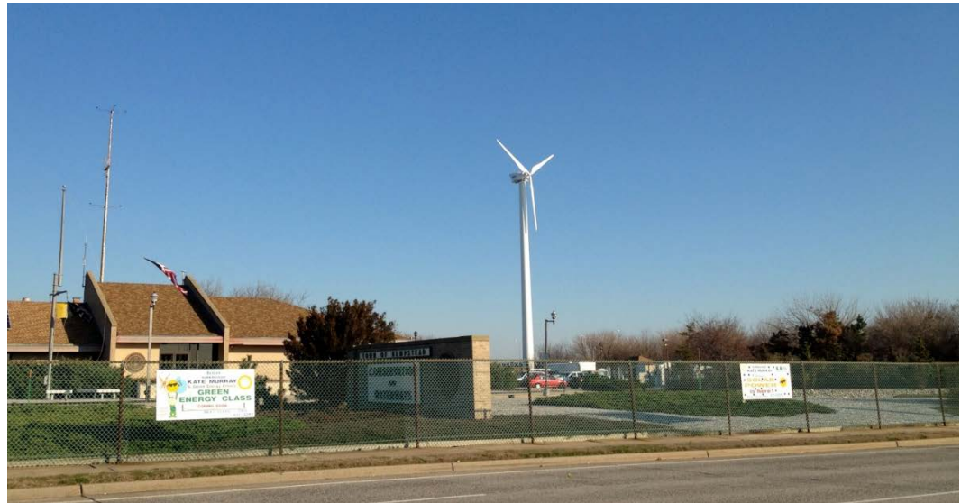
Northwind 100, 100-kW wind turbine; Hempstead, New York Photo courtesy of the Town of Hempstead, NREL 28963
