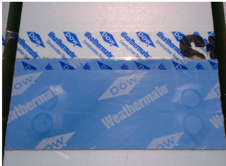
Figure 14. Example termination tape offset high on butyl tape
