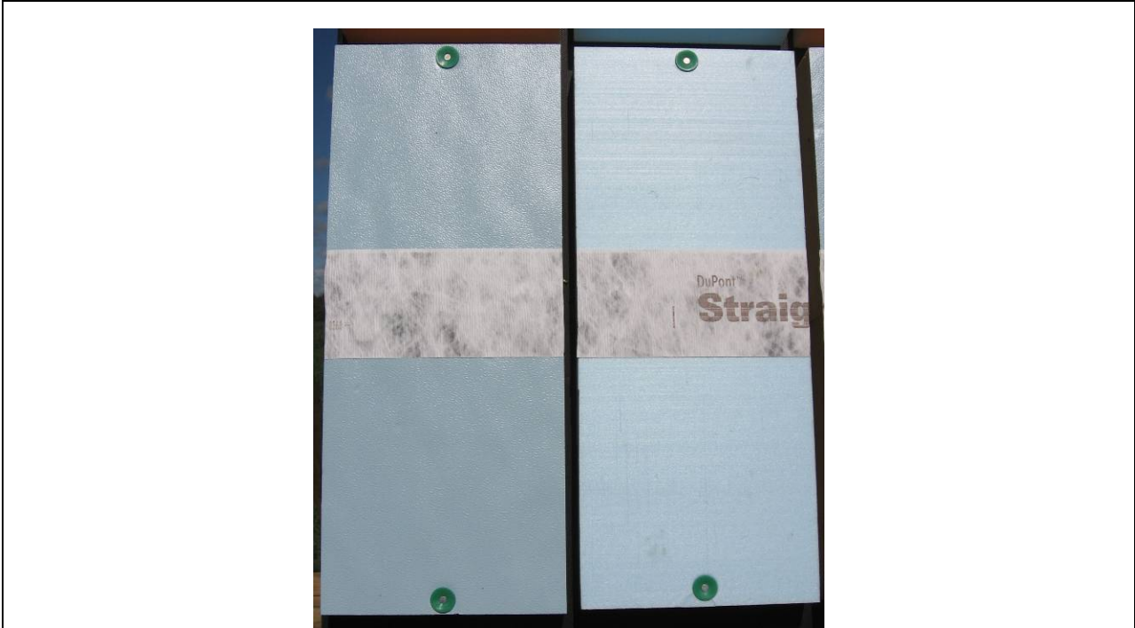
Figure 31. DuPont Straightflash tape on ffPIC (left) and XPS (right)
