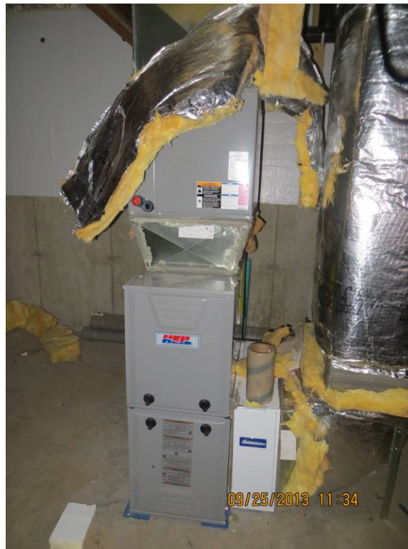
Figure 17. Air sealing around the air handler compartment
