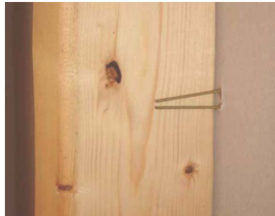
Figure 3. SIS staple missing the stud
