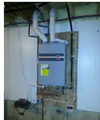
Figure 14. Condensing tankless water heater
