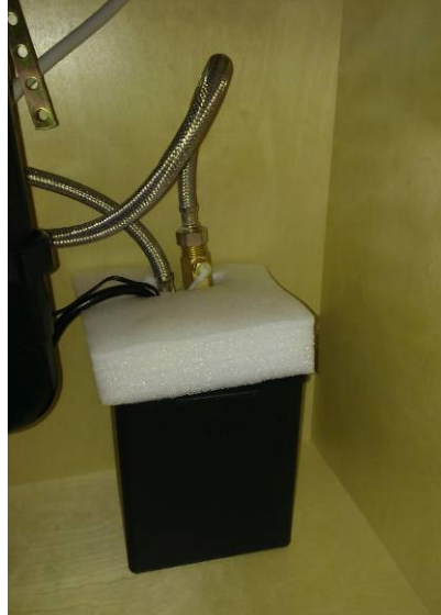
Figure 19. On-demand recirculation pump installed at furthest fixture
