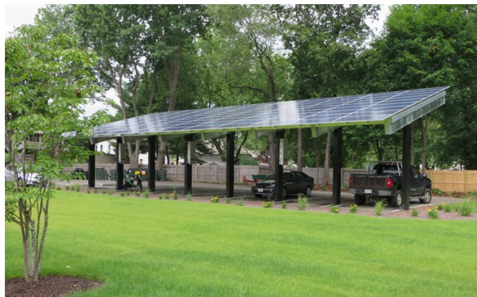
Figure 2. Above the parking area, a 30-kW PV array provides electricity to the building
