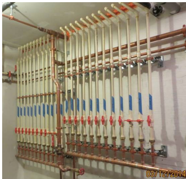
Figure 15. Hot and cold water manifolds in the mechanical room. Copper hot water piping was ultimately insulated; chlorinated polyvinyl chloride (CPVC) piping was not.
