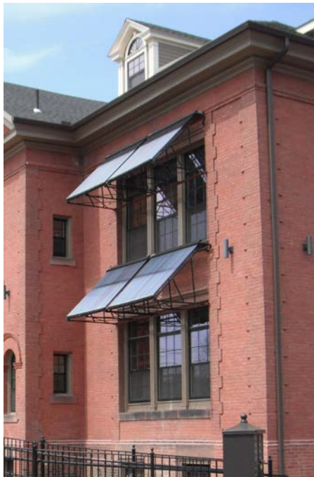
Figure 8. Evacuated tube solar collectors mounted as awnings over south-facing windows
