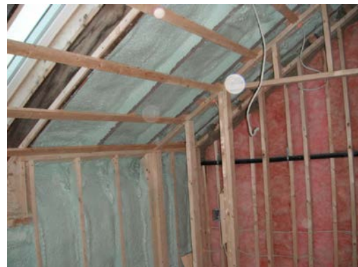
Figure 6. Wall and roof insulation on top floor. Fiberglass insulation is for sound control between rooms.
