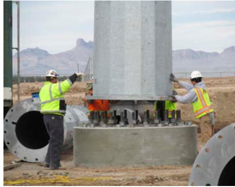
Construction crews secure the next section of the Saguaro line structure that is part of the ED5 substation upgrade. Photo from Ralph McCracken, Western Area Power Administration
