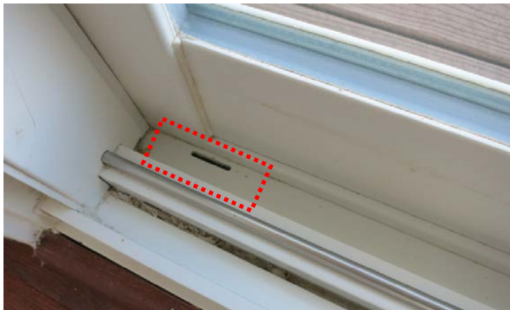
Figure 40. Sliding glass door air leakage at weep hole (door unit)
