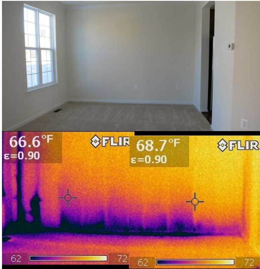
Figure 54. Second-floor living room leakage pattern over garage, Unit 6706, location D
