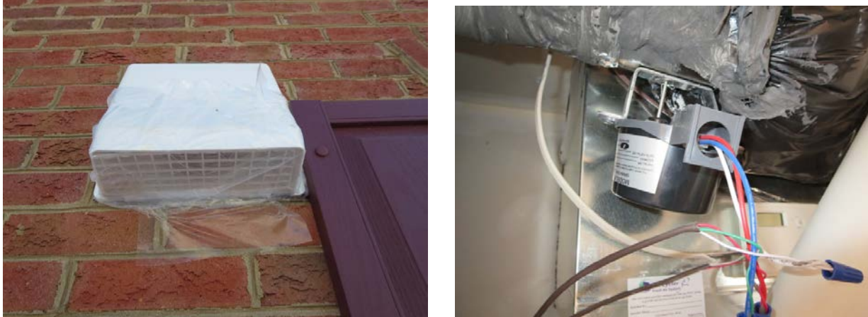
Figure 21. Outside ventilation air intake; motorized damper at air handler
