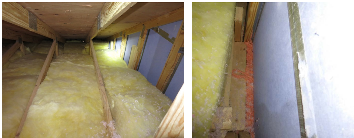
Figure 57. Vaulted attic and separation wall conditions, Unit 6704
