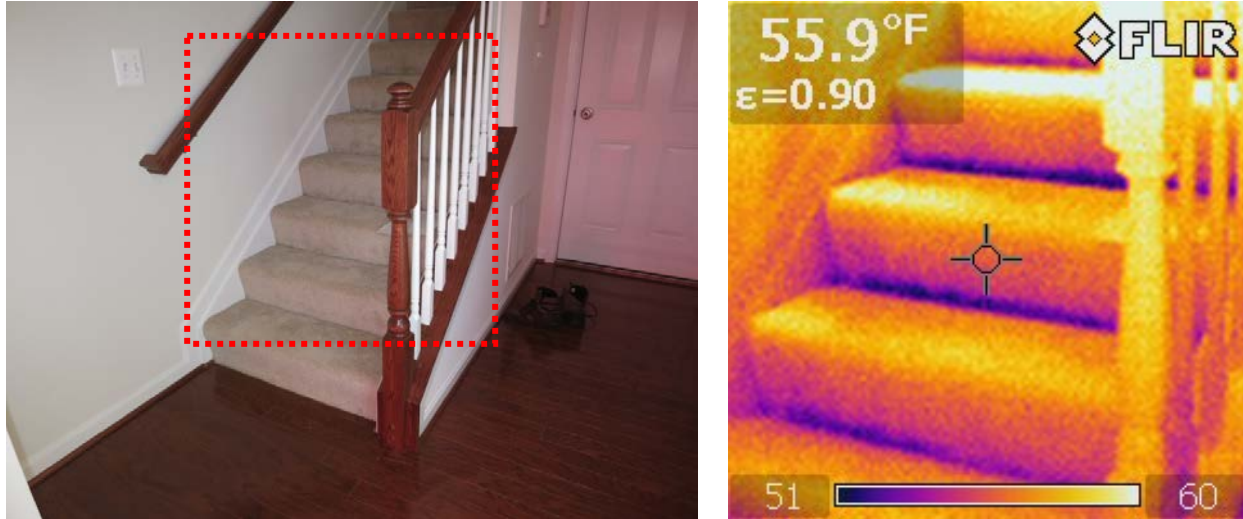
Figure 48. Air leakage at stair tread-to-riser joints, location (A)
