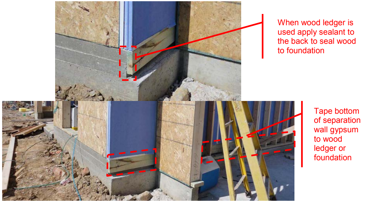
Figure 14. Wood ledger condition at area separation wall
