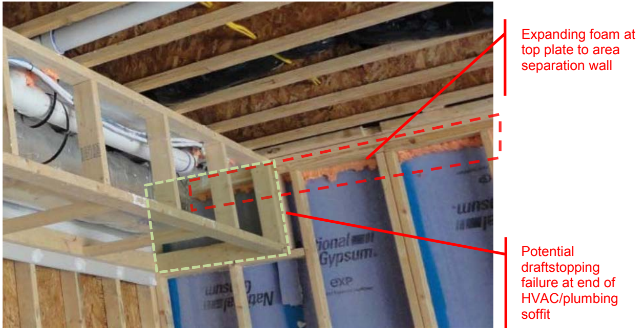
Figure 12. Expanding foam at garage, top plate to area separation wall
