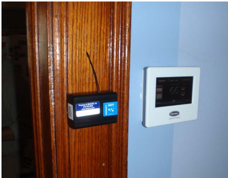
Figure 9. Wireless temperature and RH sensor at the thermostat in Test House 2
