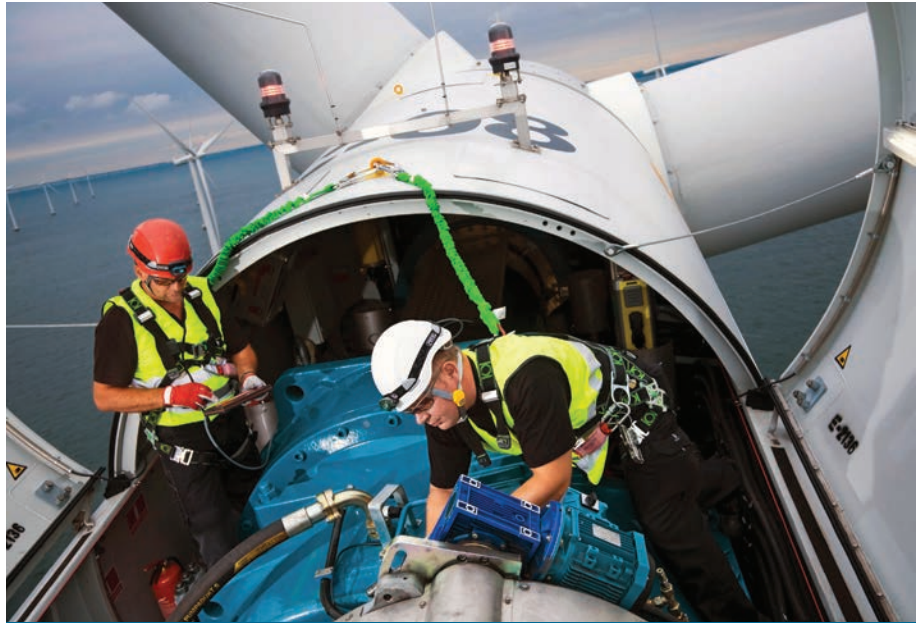
Two engineers working in the nacelle of a Siemens offshore wind turbine. Photo from Siemens
