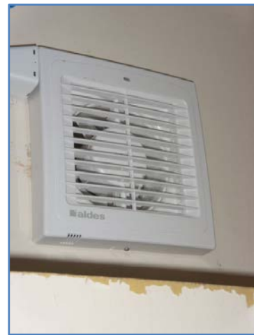
Figure 45. Interior exhaust fan grille
