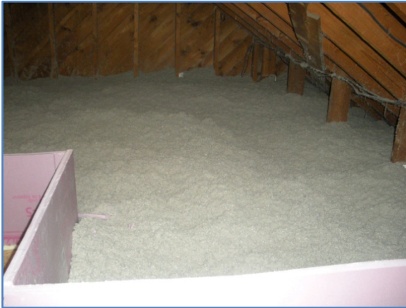
Figure 14. Insulation baffles at edge of new storage area
