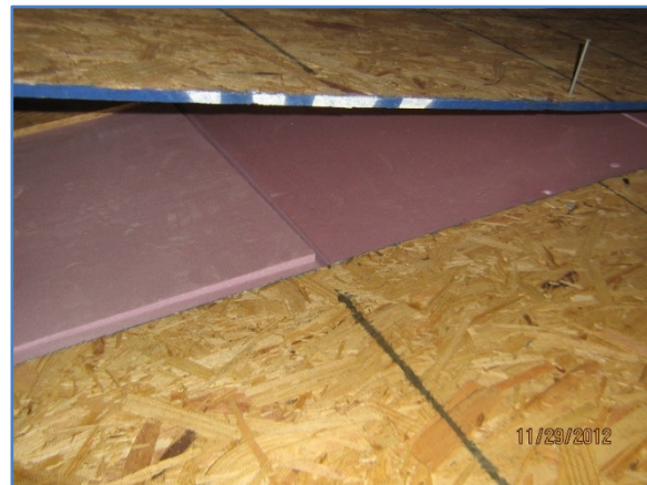
Figure 13. Wood sheathing installed over the foam board to maintain an attic storage area
