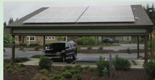
Solar photovoltaic panels installed on low-income tribal elder housing units in Oregon offset 25,231 pounds of carbon dioxide emissions—the equivalent amount of carbon dioxide absorbed by 299 trees—in August 2014 alone, and provided 100% of the electricity used by the complex in the summer months. Photo from Grand Ronde Tribal Housing Authority, NREL 31794
