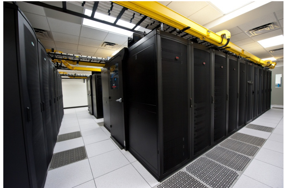
NREL Data Center Storage Arrays NREL PIX #18784
