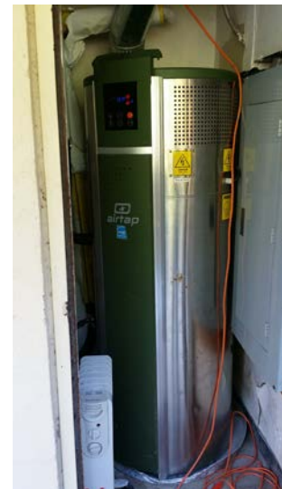
Figure 15. In a less-than-ideal situation, an electric space heater was placed next to a heat pump water heater within an apartment because the unit was overcooling the living space.
