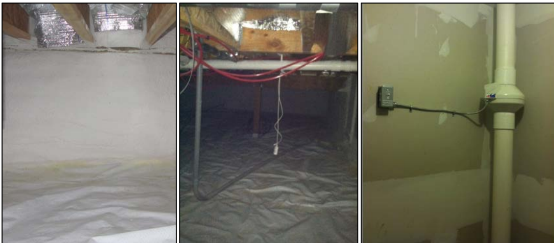
Figure 3. Crawl space insulation (left), vapor barrier (center), and vent fan (right)
