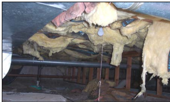
Figure 2. Vented crawl spaces often have poor insulation, no vapor control, and unsealed mechanical ductwork.
