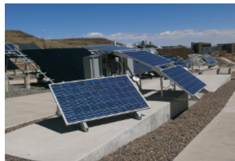
Figure 3. PV modules with micro-inverters installed at NREL. Three PV modules are south-facing, with tilts of 10°, 25°, and 40° from the horizontal. A 4 th PV module is tilted 40° and faces 30° west of south. A 5 th PV module (not shown) is installed on a nearby two-axis tracker.
