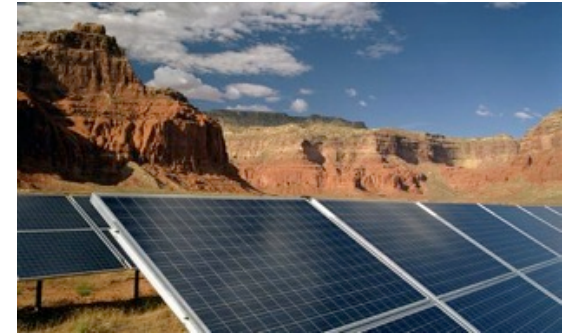
Photo by Warren Gretz, NREL 08024
