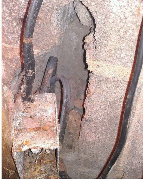
Figure 25. Abandoned basement receptacle at CMU wall
