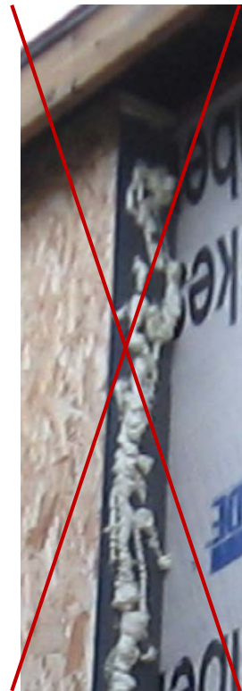
Figure A-3. Do not apply spray foam to panel edges as sealant in freezing weather conditions
