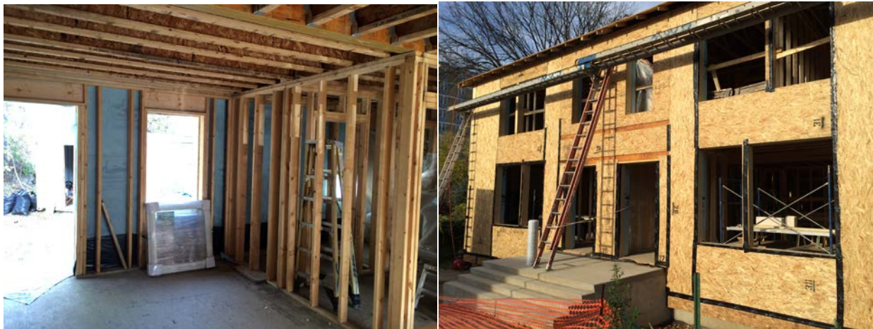
Figure 9. Wall construction—the 2 × 6 frame wall with air barrier membrane (blue) visible (left); the SIPs installed (right)
